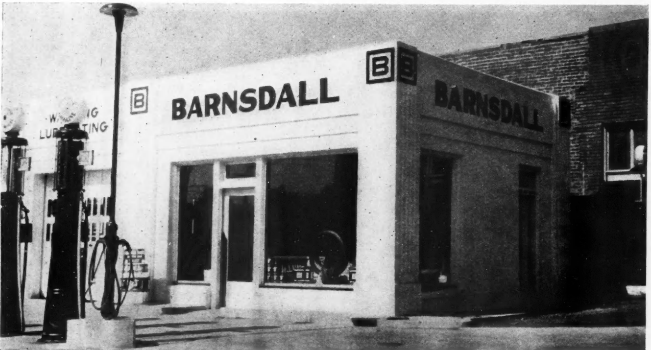
AT THE TOP OF THE PAGE, the obsolete "horse-and-buggy" type station is shown before a $4000 modernizing job changed it to the attractive and efficient service station pictured in the lower illustration. Increased business justifies such remodeling projects.
