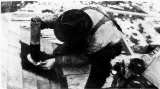
JOURNEYMAN PLUMBER preparing roof joint with tallow before wiping lead flashing to lead vent pipe.
