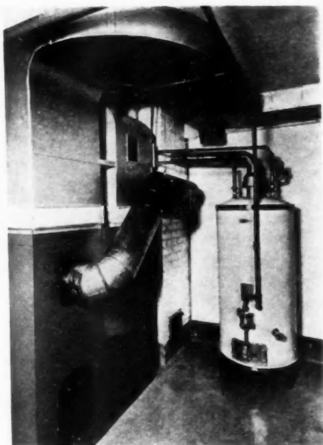
CLEAN AND CAREFREE COMFORT is made possible by the gas-fired winter air conditioner and automatic Monel metal storage water heater with a capacity of 45 gals.
