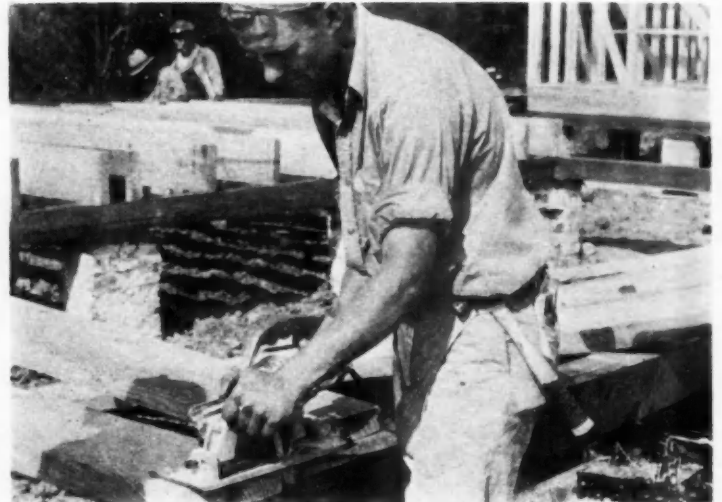
POWER SAW as shown above speeds construction job and assures square cut and accurate fit. The 6 x 6 timber sills are termite treated; the houses are set on brick piers one of which can be seen here.
