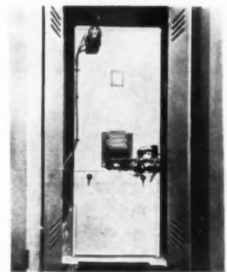
GAS FURNACE in closet.
