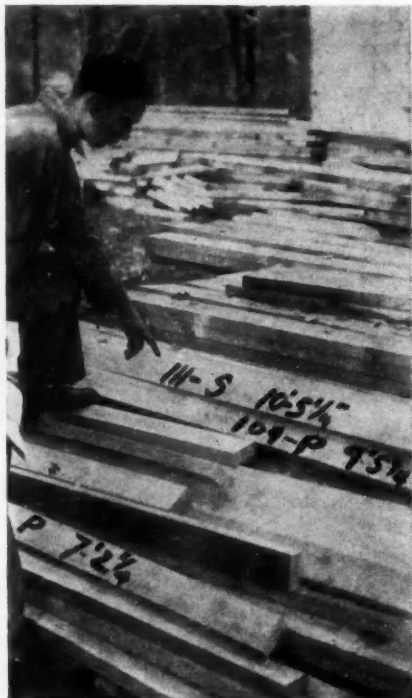
AS framing members are cut they are marked with house number and size.
