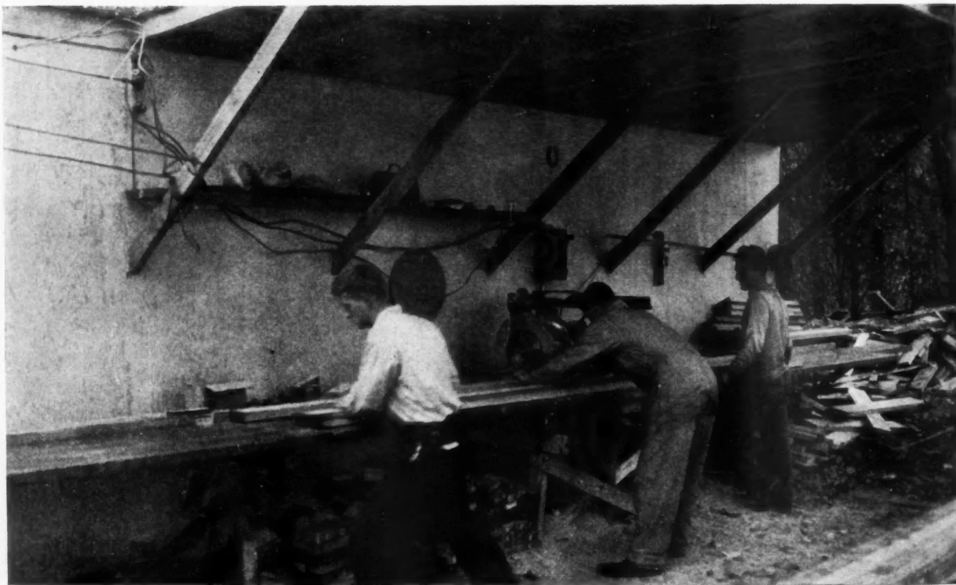
CREW consisting of saw operator and two young helpers easily cuts framing for one house a day. Pieces are numbered, stacked and delivered to site as needed by light truck.
