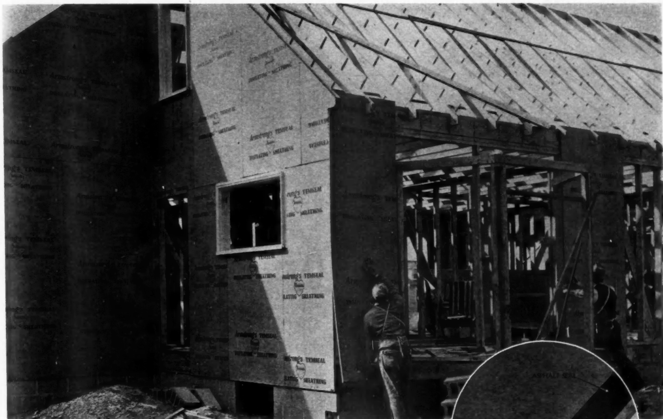
Applying Temseal Sheathing is a quick and easy operation, as this illustration of the MacFarlane residence, Mt. Clemens, Michigan, shows. Hubarth & Schott Company were the lumber dealers who supplied the material; Wolverine Shingle & Lumber Co. of Detroit, Michigan, were the wholesalers.
