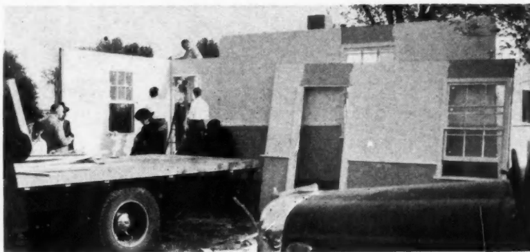
10 A.M.: First sections of Precision-Built, Jr. house at Morrisville, Pa., are set into place. Henry Palmer of Langhorne, Pa., builder.
