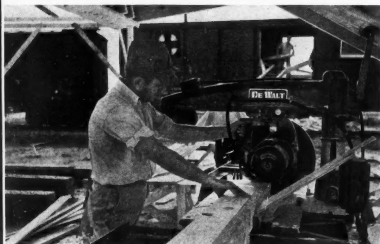
DIRECT from freight car to saw is system used at Camp Peay, Tenn., where 24 saws are set up under one shed 600 feet long.
