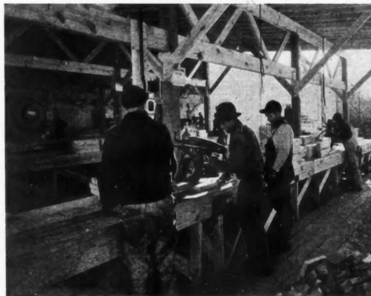
TWO-SAW HOOKUP at Fort Meade, Md., used by Consolidated Engineering Co., in the cutting of collar beams, knee braces, canopy braces and other items needed for this particular defense job.
