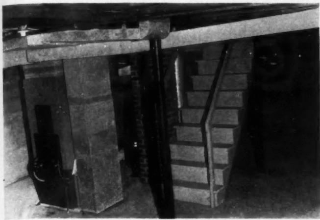
GREEN ACRES houses are equipped with oil-fired winter air conditioning unit of unusually efficient type.
