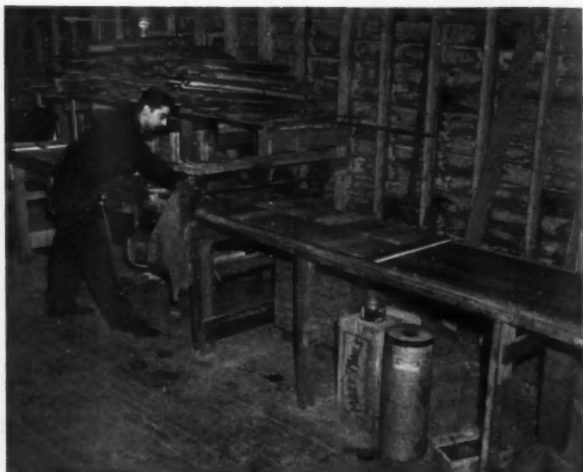
PANELS are built on a table with a steel top. Insulation board, building paper, and red cedar shingles are applied in that order. The shingle tips are trimmed by a small circular saw.
