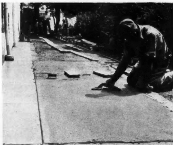
FIRST floating forces color mixture into concrete surface. Should be discontinued as soon as surface becomes wet.
