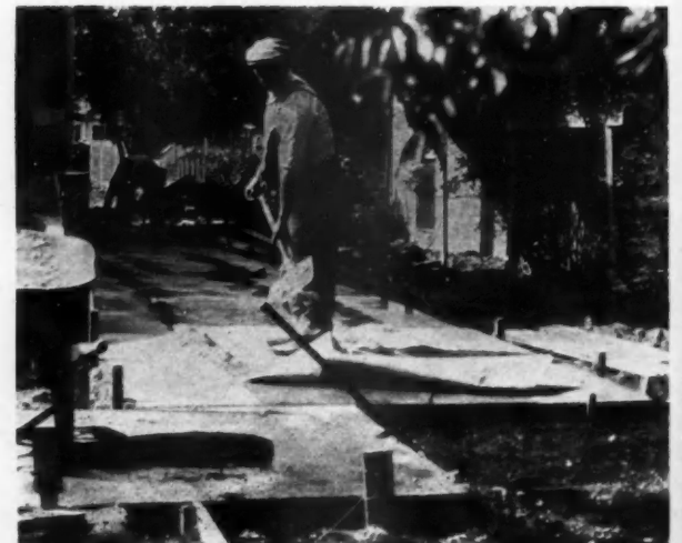
CURING concrete sidewalk by covering with waterproof curing paper; particularly recommended for colored surfaces.
