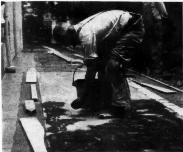
CONCRETE slab is screeded to proper elevation and excess water removed. Dust-on color mixture is then spread uniformly not less than 125 lb. per 100 sq. ft.
