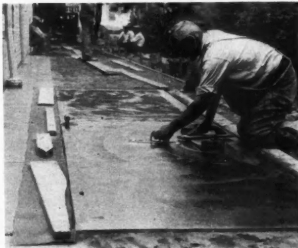
STEEL troweling to a smooth surface. Final troweling should be delayed until water sheen produced by floating has practically disappeared from the surface.
