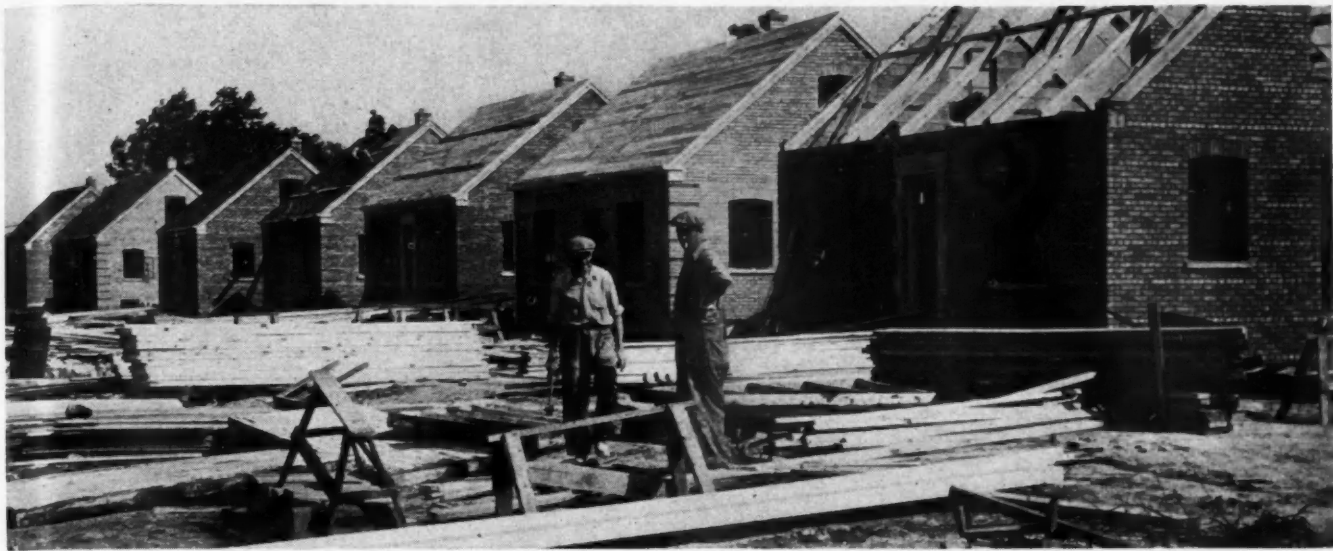
ON-THE-JOB view at Mills' Westbrook development of war housing near Chicago; workmen splicing wood gutters in the foreground.
