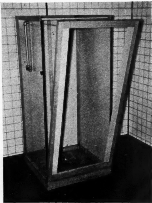
PARTIALLY assembled shower cabinet, with side and back panels attached to concrete receptor and with front assembly being set in position.
