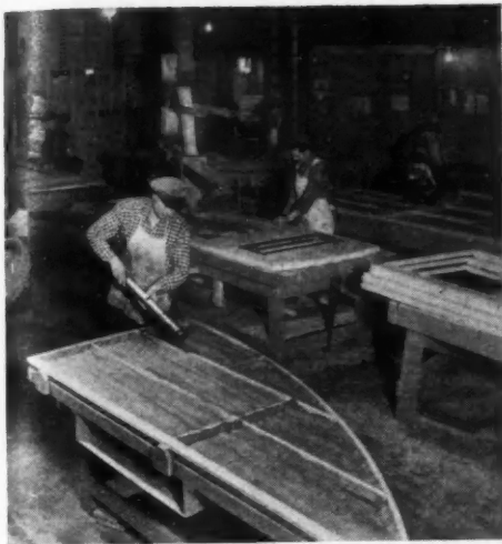
Worker above on production line is applying glue before nailing plywood over insulated prefabricated sections of U. S. Navy huts.
