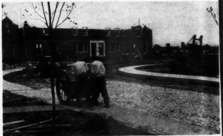
ROADS TO PEACE —Grading and paving equipment (above) helps get the war housing project of W. Thomas Buckley Building Corp., Chicago, ready for occupancy; one of the duplex apartment buildings shown.
