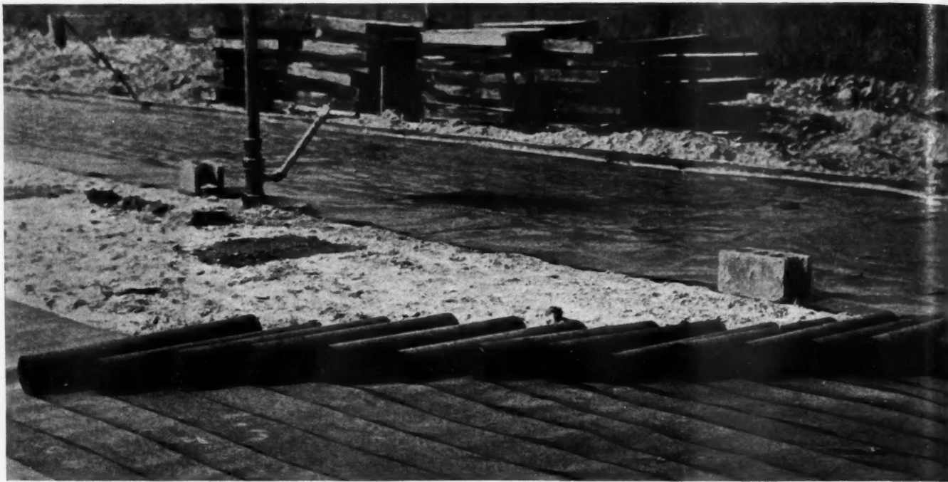
CONCRETE FLOOR SLAB was laid over this waterproof membrane consisting of four layers of 15 pound felt. Joints were lapped with hot tar.
