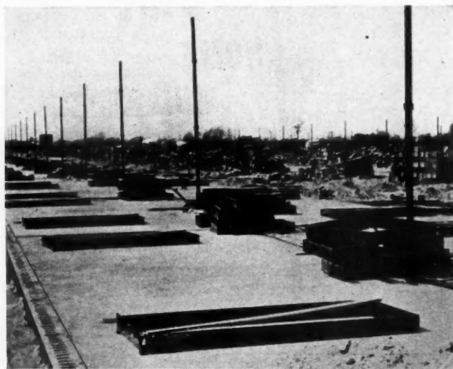
SOIL PIPES RISE from the continuous concrete slab of row of war houses at Norfolk. Shop-built plumbing assemblies were installed prior to placing of concrete slabs. Houses built under Title VI.
