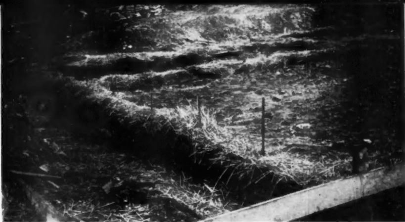
FRESHLY poured foundations are protected against freezing by covering with waterproof building paper and then with a layer of dry straw or hay.
