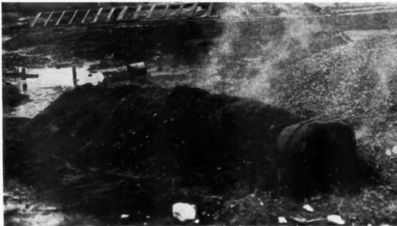
SAND and gravel can be heated by piling it over a metal culvert pipe or other improvised heater in which a fire can be kept going.
