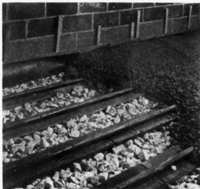
RADIANT heating installation going into a recently completed war plant. This system with heating coils buried in 6-inch floor slab holds promise of wider post-war commercial and industrial use.
