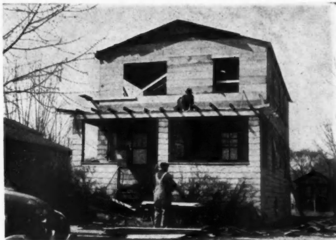
THE present roof is left on until the walls are up and a temporary roof laid to keep weather out.
