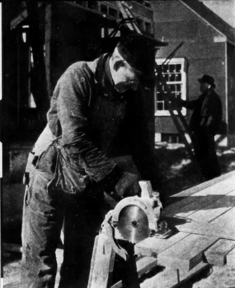
IT takes about a tenth of the time to cut studs with a power tool
