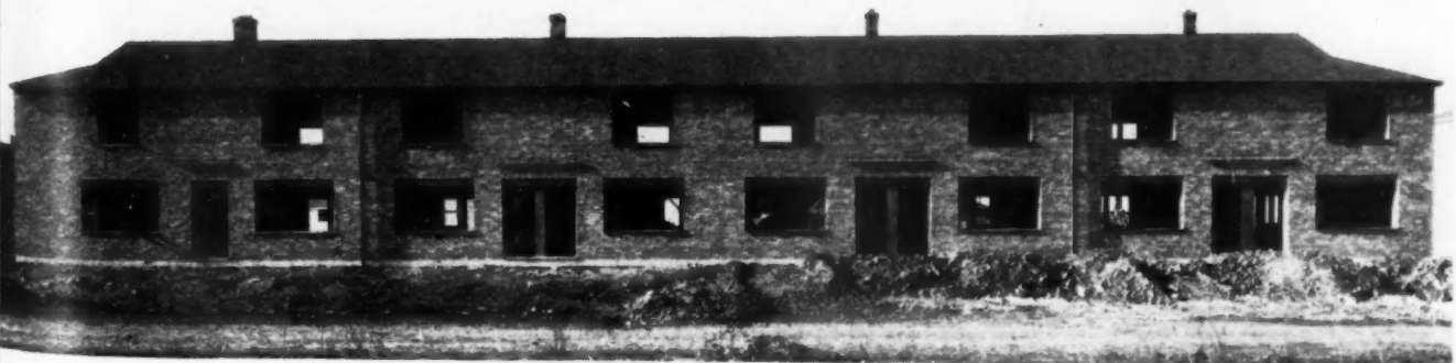
VIEW of one of incompleted eight-family apartments. Wide window openings provide for plenty of daylight and fresh air.
