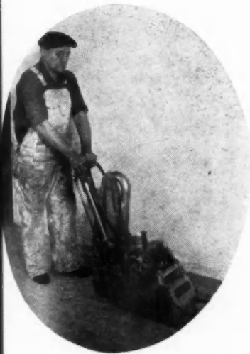
A PAIR of sanding machines make short work of floors after all else is done.
