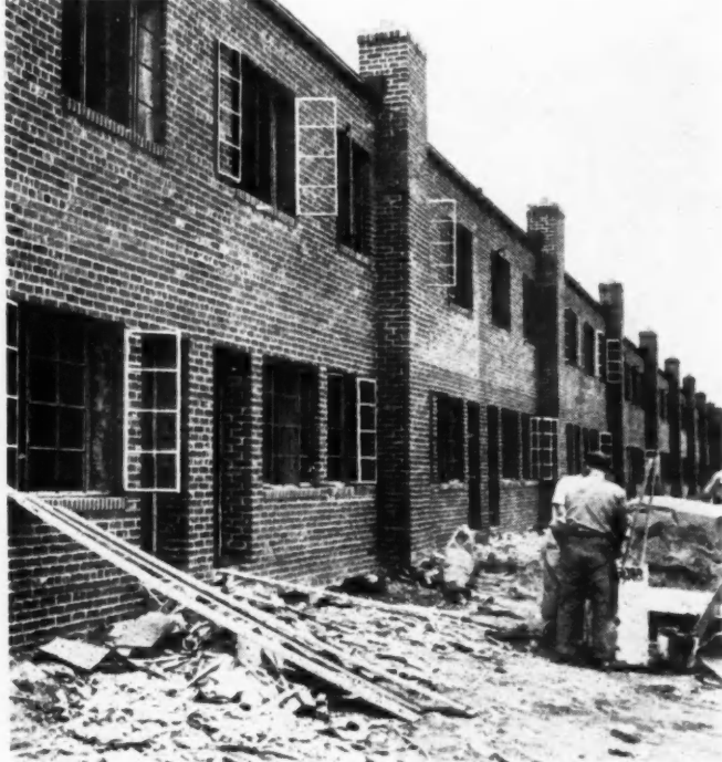
LARGE window areas and a second entrance are at the rear of each unit, overlooking a 20 x 35-foot garden or lawn space.
