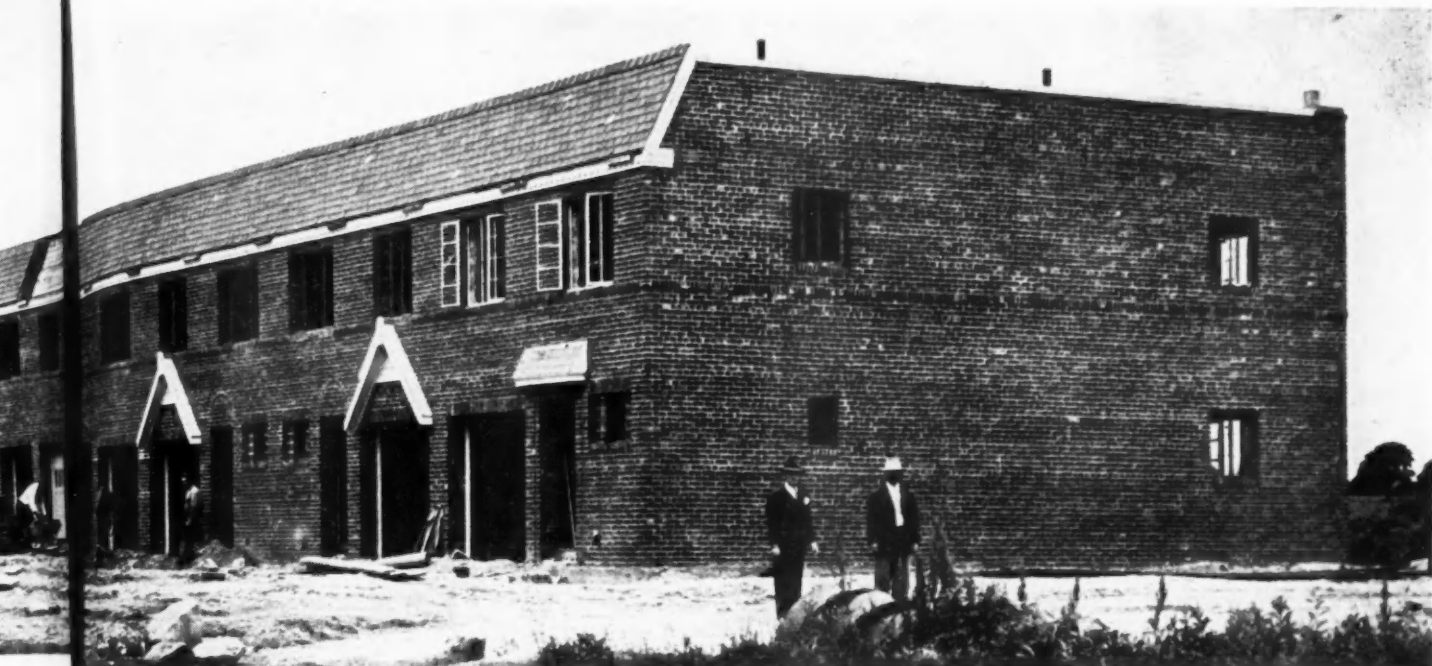
NEARING COMPLETION, the first row of eighteen homes in the Rossbach project is a complete sell-out to war veterans.
