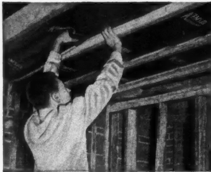
Installing light, flexible KIMSUL* in a CAPITOL PROPERTIES, INC. home. It is easy—just cut KIMSUL to desired length, expand it, and staple to ceiling joists.
