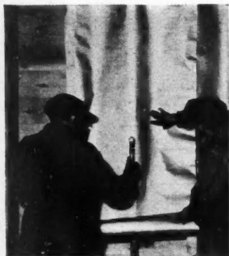
AB27108—Workmen above are installing Sisalation on studs in new house construction. This product is an effective insulation against winter cold and summer heat in addition to serving as a moisture barrier. It is a product of the Sisalkraft Co., Chicago., which also makes copper-armored Sisalkraft.
