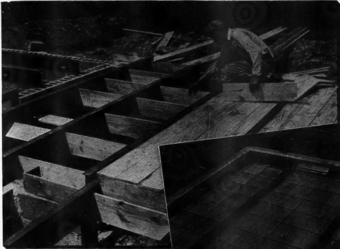
Spreaders are placed about 30" to 36" centers. A few nails hold the four 8" form boards in place. The boards can be used later as roof sheathing. Concrete will encase ends of beams to provide a fire stop and support for a bearing partition.
