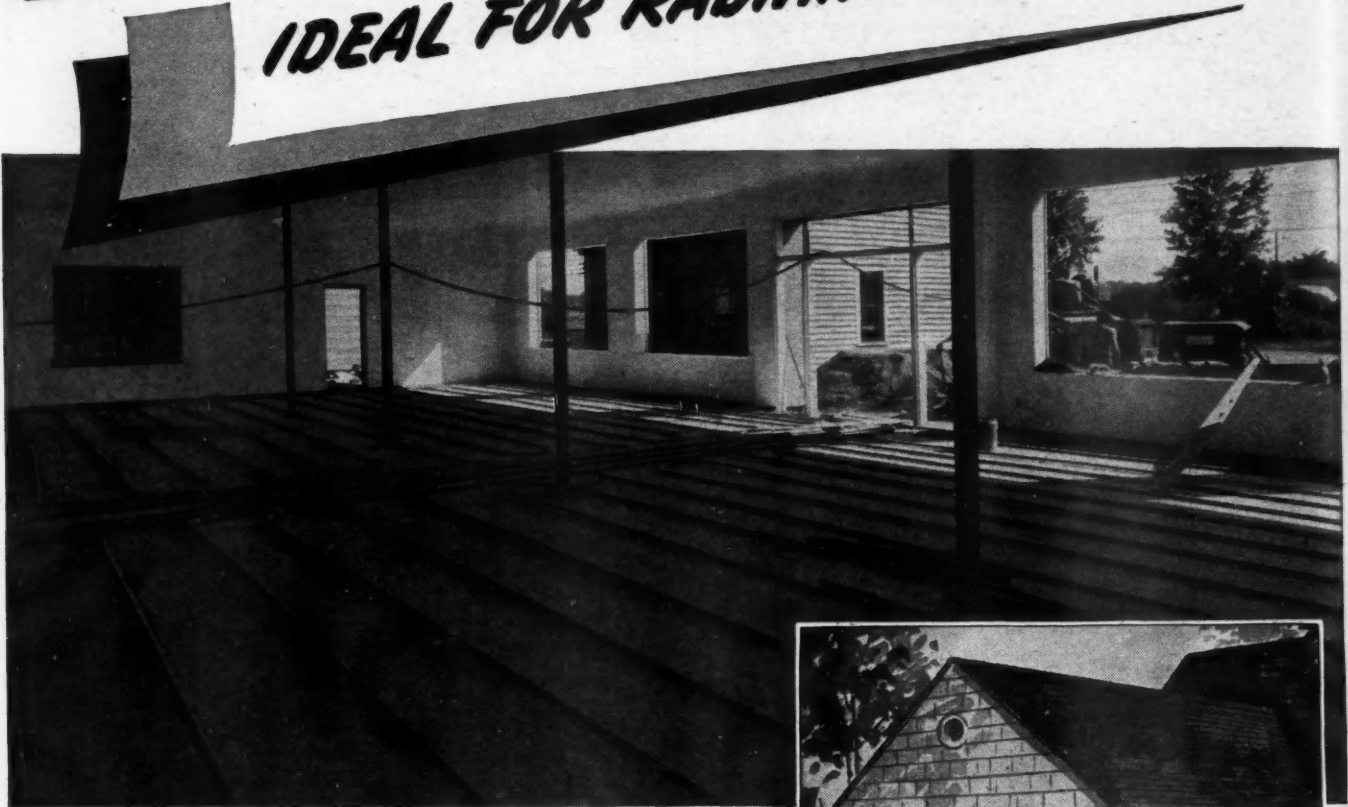
* Radiant Heating Coils resting on Zonolite concrete ready for topping of ordinary concrete.
