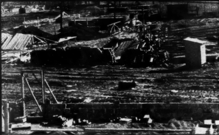
CONSTRUCTION methods are completely conventional. Notice the solid brick and masonry wall well under way in the foreground.
