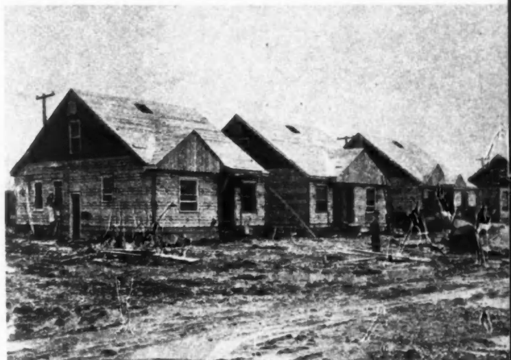
PARTS for these houses under construction were preassembled in off-site workshop on metal jigs which permit wide variation in design.
