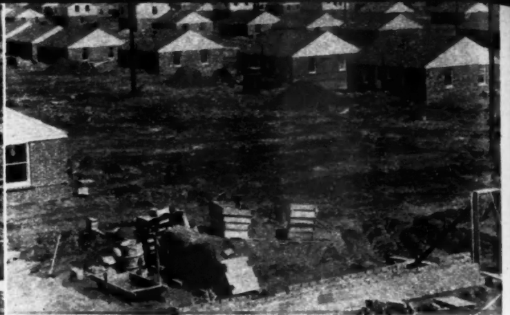
BECAUSE sewer lines were not available, septic tanks were required. Installation is being made in the houses in foreground.
