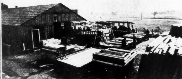
ASSEMBLING on jigs set up outside the workshop which houses more jig tables. Lumber is brought here by roller conveyors.
