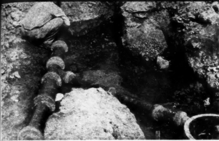
HERE workman is making final hookup to septic tank. Type of soil and drainage are important factors in installation of tanks.
