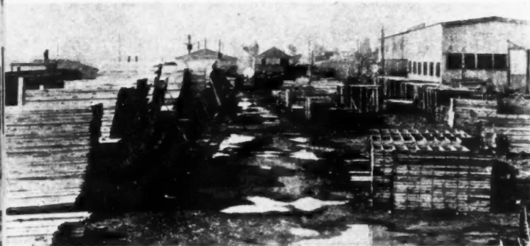
VIEW OF off-site fabricating operations. Note the narrow gauge track on which a cut-off saw can be moved to lumber piles.
