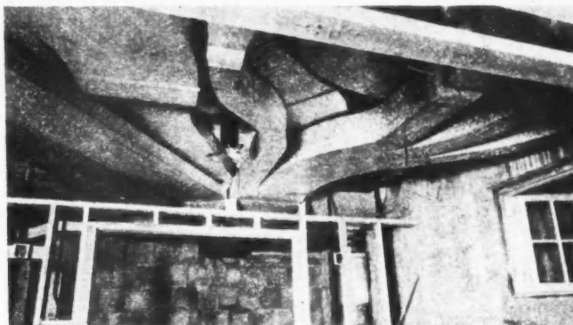
GOOD duct work is essential.
