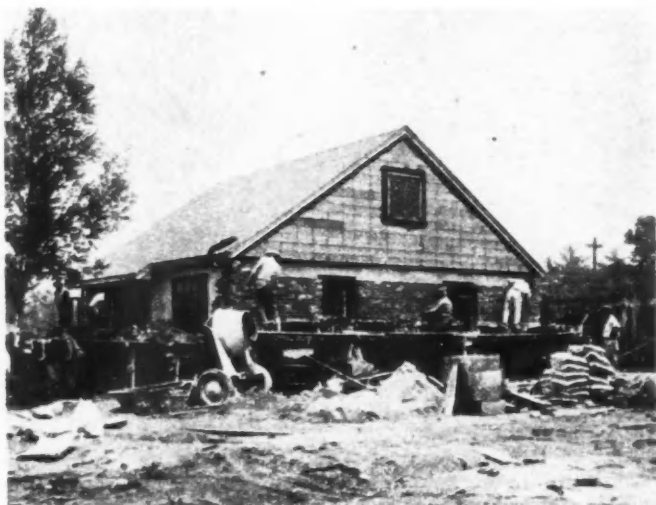
BRICK veneer being applied to face of concrete walls. Roof of frame.
