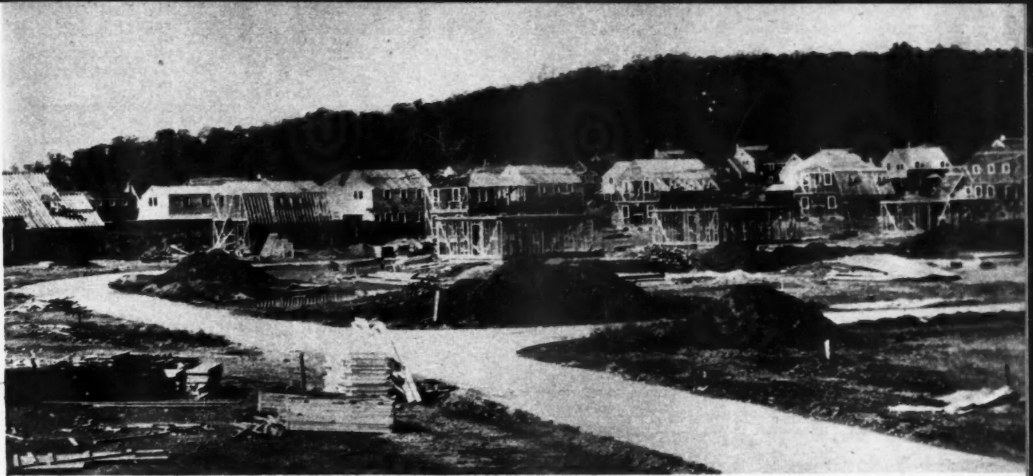
A PANORAMIC view of Levitt's latest deluxe housing development shows the impressive size of a mass operation
