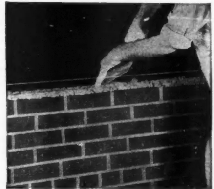
Mortar for this bed joint was spread out on the wall too far.
