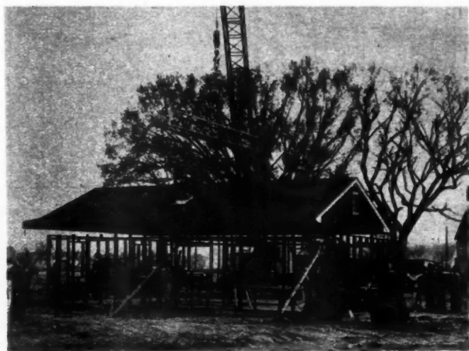
THE roof section is trucked from the fabrication shop to the house site and lowered to the steel frame by a heavy crane with a 60-foot boom. The roof is then welded to the wall sections
