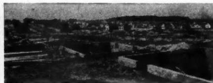
ADJUSTABLE steel posts were used in basements of this 400-home Heslop project
