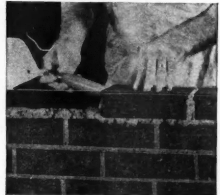
So the mortar dried out too much before the next course of brick was placed on top of it.
