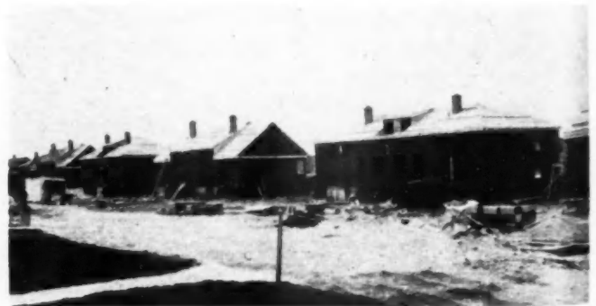
REAR view of a row of duplexes that are ready for brick veneer
