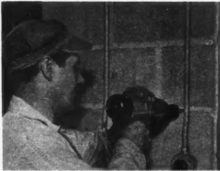
A HOLE in concrete can be drilled in seconds with a carbide-tipped drill
