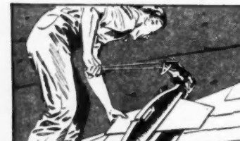
6. Cutter Speeds Application —When shingles must be cut to fit around valleys, dormers, along the rake, etc., a shingle cutter does the job easily, quickly—right on the roof.
