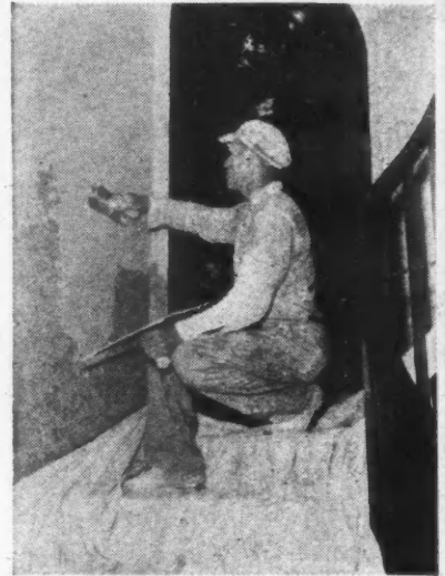
WORKMAN applying a thin coat of new bonding plaster to rough wall surface
