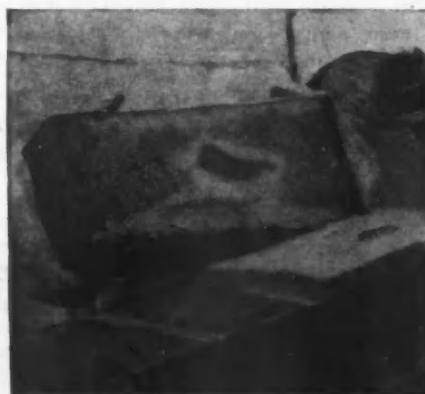
Therefore the mortar did not stick to the top brick. A good bond was not secured.
