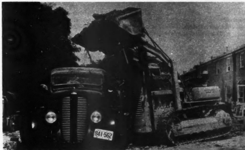
TRACTOR-SHOVEL combinations offer maneuverability and low cost necessary to dig basements quickly and cheaply. This Caterpillar D4 and Traxcavator shovel completes a 28x30-foot basement in four hours—and does it on only 39 cents worth of fuel. It will do other jobs equally well
