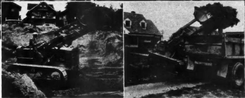
AN Allis-Chalmers HD-5 equipped with a Tracto-Shovel is shown excavating the basement for a home. This is only one of its many uses around a building site
