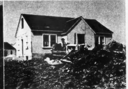
LANDSCAPING and terracing around houses is made easy with this equipment. Unit here is a Caterpillar Diesel D7 tractor equipped with a 7A bulldozer
