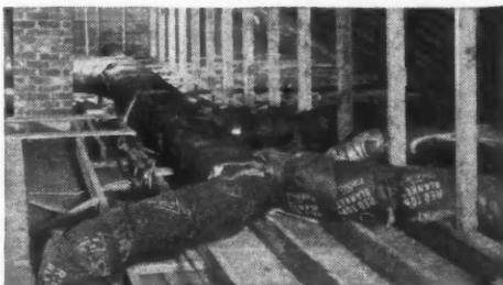
Attic view shows insulated supply ducts that connect via warm-air inlet boots to the ceiling panels below. Sealed insulation board is used to form top of ceiling plenum. Uninsulated pipe at right is exhaust for kitchen ventilating, not connected with heating system. Photograph taken before insulation was installed between joists.
