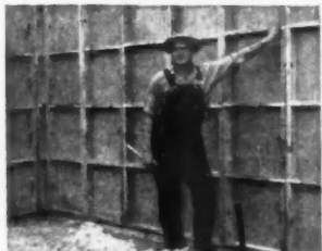
"Seven men set-up the forms for a 26' x 27' basement in one hour and fifteen minutes."—Harry G. Dehring, Carpenter Foreman, Taylor Brothers, South Bend, Indiana.
