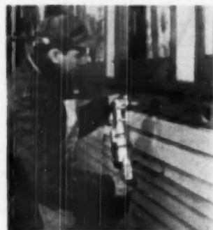
CONVENIENT handles and special bit of RAD drill aid worker installing insulation in old home
