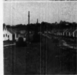
ALTHOUGH Timely Homes sublet all pavement work up until 1950, equipment shown here working in the project last fall was on the list for purchase by this builder so it would be on hand for use in completing 500 or more homes in 1950
