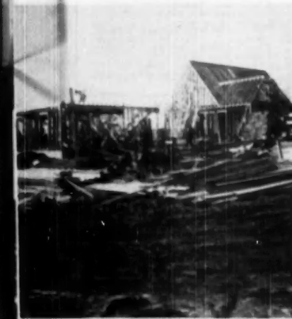
NOTE steep pitch of roof necessary to conform to local code demanding minimum 22 feet from top of first floor to ridge
