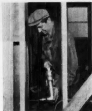
WITH right angle drive in low position, electrician drills holes in difficult spot for installation of electrical conduit
