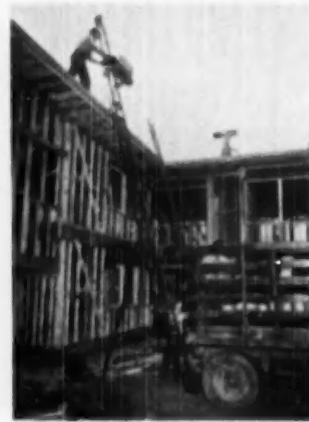
CONVEYOR in action on project. Machine is capable of lifting 14½ tons per hour
