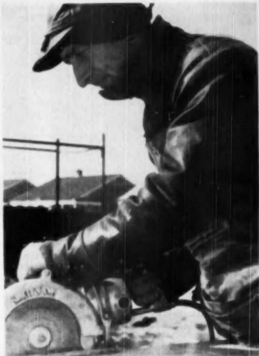
POWER hand saws are big time-savers in the current Robbins project, where a system of materials handling and rough framing keeps them almost constantly in use. Saw shown here is made by Skil saw
