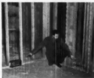
BEDROOM register location shown above should have been on wall at right where narrow space between openings precludes location of furniture. Location on large wall at left, dictated by framing, can cause housewife annoyance when planning bedroom furniture arrangement
