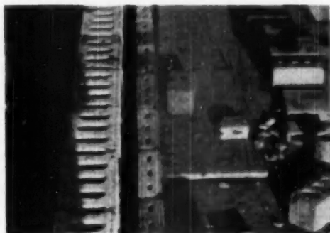
CONCRETE block wall, consisting of parallel rows of eight- and four-inch blocks with 2-1/2 inch cavity ready to receive 1:4 vermiculite mix.
