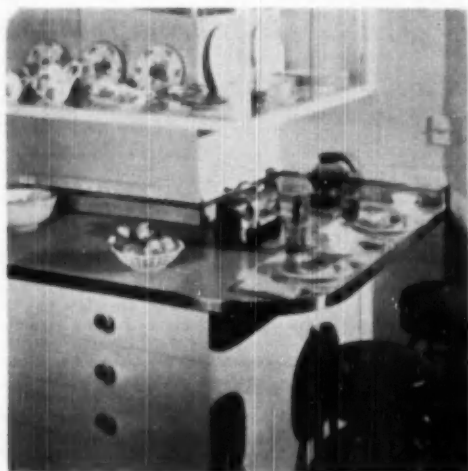
MOLDINGS enclose electrical circuit and with frequently spaced outlets provide maximum convenience for use of countertop
