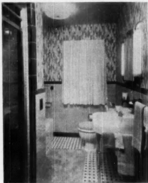
AN electrical heater installed in the tiled wall of this bathroom furnishes radiation and convection heating for quick warmth
