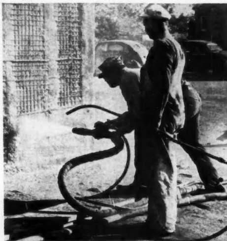
AFTER sand blasting all loose and weather beaten masonry from the exterior, a new finish of concrete was applied pneumatically. This varies in thickness from three to seven inches
