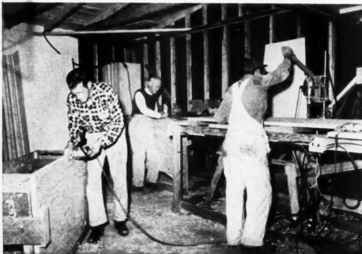
INDOOR shop of cutting yard. workman at left uses door plane; at right, door is drilled for lock hole, and third workman cuts butts with router. Cutting yard is 100 by 200 feet
