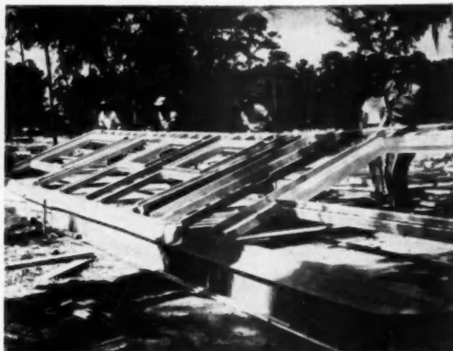
COMPLETE wall sections are assembled on a concrete slab, using precut members and fabricated window and door bucks. After wall is raised, plumbed and corner-braced, next building is ready
