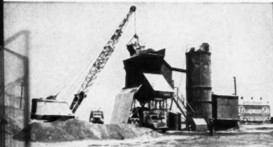
BATCH PLANT measures materials, dumps dry mix and water into trucks. Materials firms installed two batch plants at job
