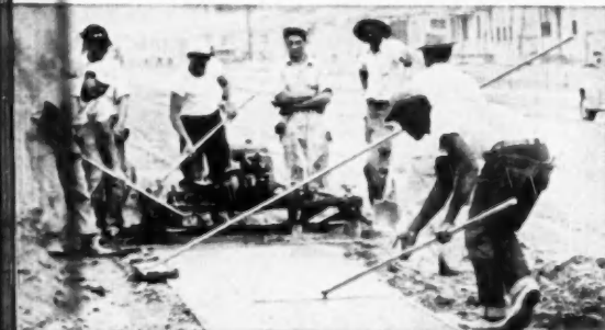
VERSATILE TOOL in action here tamps concrete, puddles and compacts it, rods it off. Machine is pulled over walk by two men
