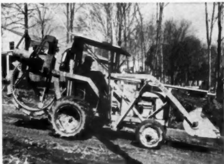
COMBINATION TRENCHER and front end loader. This machine is used for digging foundation walls, footings, sewer, water lines
