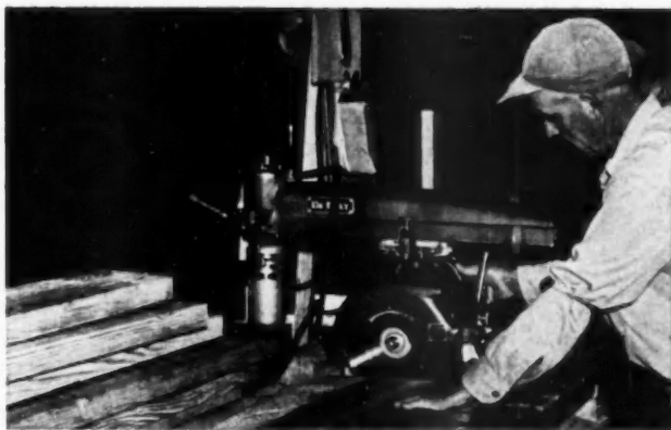
RADIAL arm saw, placed at one end of the long marking table, is kept busy almost continuously. All plates (base, raiser and top) and studs are cut to length for 30 buildings at a time. This precutting system saves company over 15 per cent on materials
