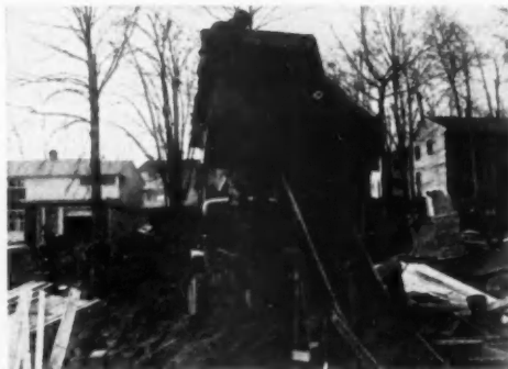
HIGH DUMP BODY mounted on a G.M.C. 6 x 6 chassis unloading cinders on metal chutes at building site, helps speed completions
