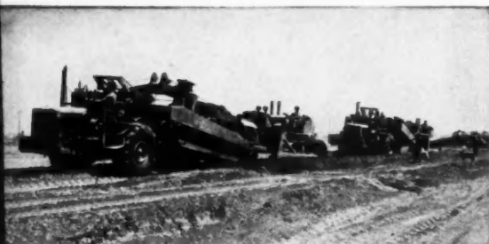
SELF-LOADING machines, pushed by tractors, are important equipment in the Lakewood Park project's extensive grading
