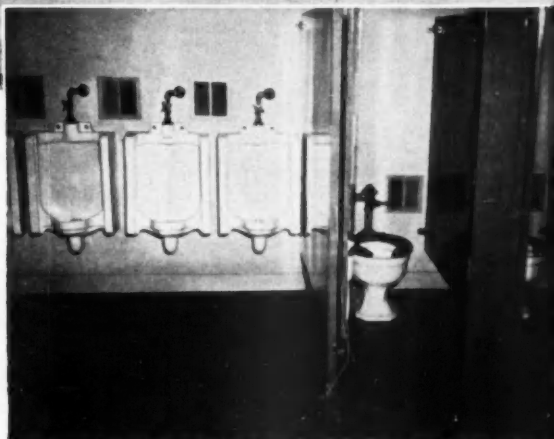
Section of Cold Spring School wash room showing the batteries of Richmond Delton Washout Urinals (Plate No. G-353) and the Richmond Spaulding Syphon Jet Water Closets (Plate No. G-220).
