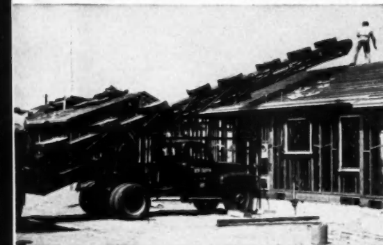
ESCALATOR delivers bundles onto endless belt which carries them in steady stream to ridge of roof, ready for application. Belt is reversible, to permit the return of surplus bundles
