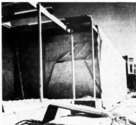
COMPLETE CANVAS enclosures, with steam heat, will protect masonry materials when temperatures are below zero
