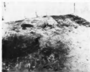
"PROBLEM FLOOR": factory trucking area before Roc-Wood application
