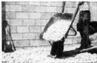
1 Compact soil thoroughly to prevent unequal settling of floor slab. Then add a coarse granular layer (usually 6 in. thick) of either slag or crushed stone or gravel, 1 in. or larger in size.
