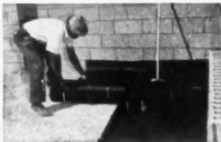
3 Before asphalt cools apply layer of 15-lb. roofing felt, with edges well lapped. Mop with hot asphalt, place second layer of felt at right angles to first layer and mop with asphalt.
