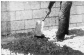
2 Compact granular fill. Cover with layer of stiff concrete at least 1/2-in. thick to provide smooth surface for moisture barrier. When the concrete hardens mop surface with hot asphalt.
