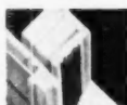
2 1/2" outside sheathing and 1/2" lath and plaster on 2 x 4's—and Superior full width jamb
