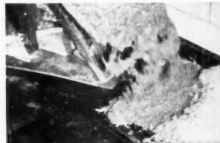
6 Place carefully proportioned concrete over dampproofing and insulation. Add metal reinforcing weighing at least 40 lb. per 100 sq. ft., positioning it 1 1/2 in. from top of 4-in. slab.
