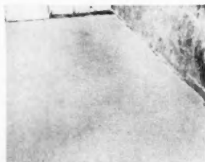
NEW SURFACING with Roc-Wood on same floor. Material can be simply applied with trowel
