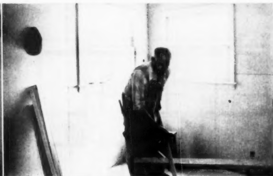
Finish carpenter can trim house as wallboard is being installed. Owners do the seam finishing
