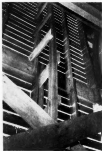
Laminated truss nailed to the center stud of the crib reinforces the end wall. Truss is 24 feet in length
