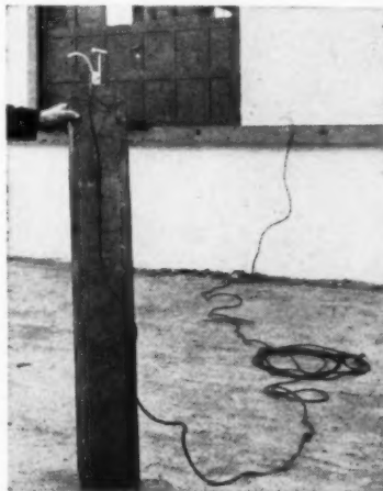
Board is placed in a spot correct in height, and a mark indicated at liquid level; as board is moved, difference between liquid and mark will show when fill is to be added or removed.
