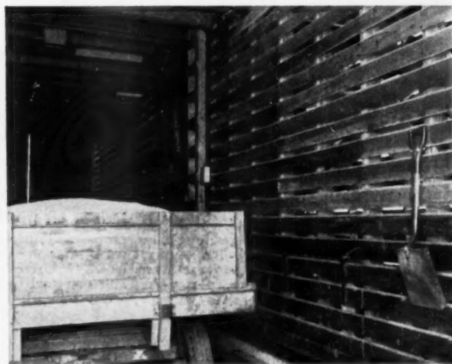
Thirteen foot drive has plenty of room for a truck. Overhead is a 3,800 bushel capacity storage bin for small grain. Elevator on the right carries grain up to bin. Capacity of the two 8x54 foot cribs is 7,200 bushel
