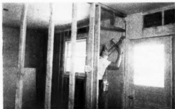
Wall board is applied to large areas. Then partitions are set in place
