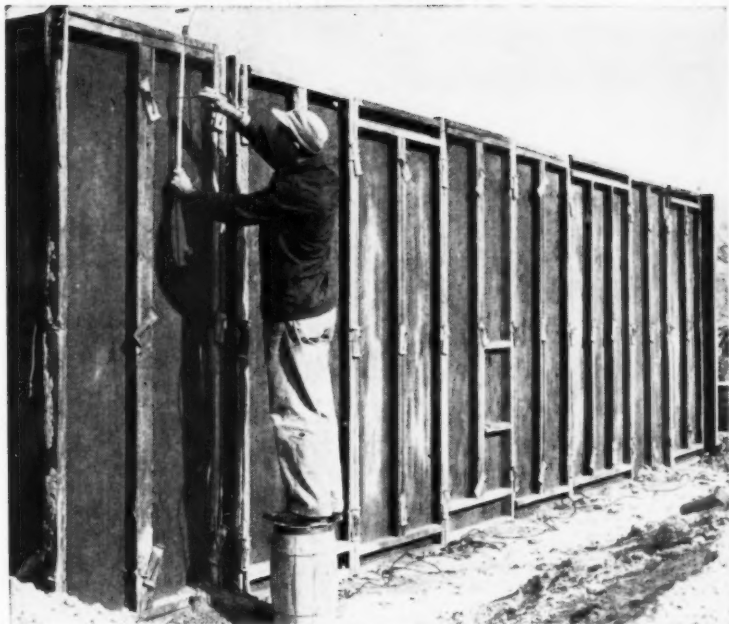
Placing nails to show correct height for concrete in forms. A level line is established by liquid, then location of nails is referred to this line by measuring with ruler
