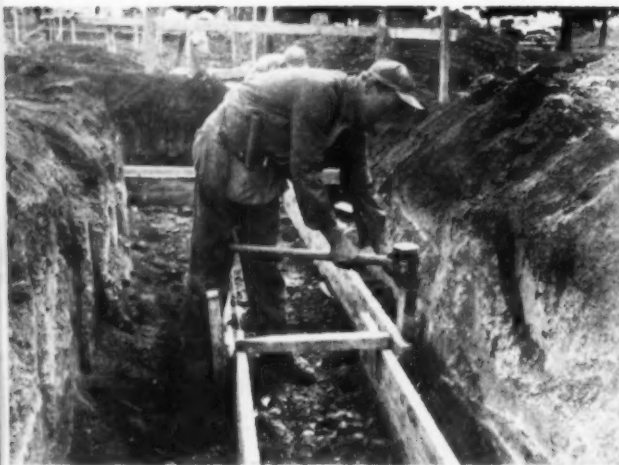
Trenches are cut wide so that men can work in them. Footing is 10x20 inches
