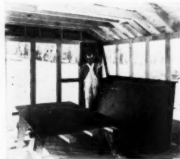
Carpenter is shown nailing a panel into place on a Lake Hotel cabin in Yellowstone National Park. He is nailing to the inside of the framework, so that the smooth side of the Masonite \frac{5}{16} inch Tempered Presdwood will be exposed. After painting, the textured side of the panel presents the appearance of canvas
