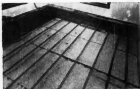
A typical floor heating coil installation. The serpentine coil is made of 3/4-inch black iron pipe on 12-inch centers. Joints are welded. Gravel fill is covered with weatherproof membrane. L-type insulation is used along exposed edges of floor. Pipes are ready to be covered with sand aggregate cement. Cement should enclose pipes with at least 1 1/4 inch of concrete over top of pipe
