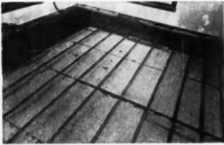
A typical floor heating coil installation. The serpentine coil is made of 3/4-inch black iron pipe on 12-inch centers. Joints are welded. Gravel fill is covered with weatherproof membrane. L-type insulation is used along exposed edges of floor. Pipes are ready to be covered with sand aggregate cement. Cement should enclose pipes with at least 1 1/4 inch of concrete over top of pipe
