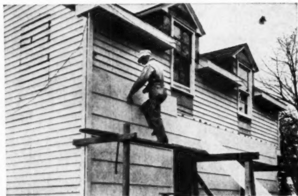
Wide-lapped plywood siding was applied directly to old section of house over drop siding; new dormers add light and ventilation
