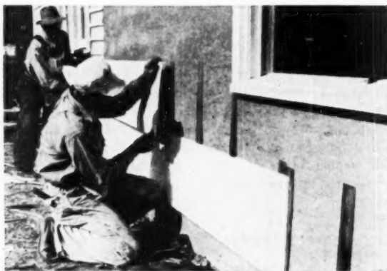
Shingle wedges were placed at nailing joints as solid base for wide-lapped \frac{3}{8} -inch plywood siding that carries out the horizontal effect of the new design
