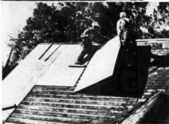
Old shingles were removed and structural plywood laid down over old roof deck as a solid base for new shingles
