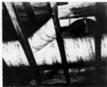
Attic installation of fiber duct: note feeder line running from supply line
