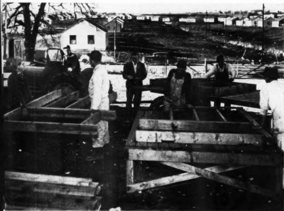
In the cutting mill yard: Material is piled in foreground, next to jig on which it will be used. Two carpenters on the jig are nailing stairwell frame together and the four pieces of ceiling joist that go with it. After frame is nailed, two handlers at left carry it to flat-bed wagons which convey it to site. Assistant superintendent (center) makes periodic checks of all jigs, cutting lists, tools and the amount of work produced in a given time. Orders are filled by matching a card index which shows everything on the wagon against the written request for material by the superintendent in the field. This way, the job superintendent can know how many houses are on hand already cut, amount of material in yard and how much has been site-delivered
