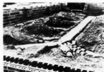
Graduated trunk and multiple "Y" feeder assembly used in auditorium zone. Feeders are made up of concrete tile joints sealed with vapor barrier sleeves
