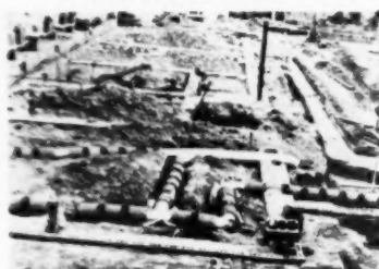
Perimeter installation serving rear section of the building. Trunk duct (right) lies under corridor. Loop and feeder ducts (foreground) are under kitchen
