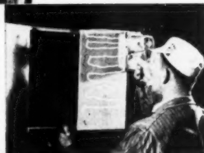
ORBITAL SANDER smooths same door in 40 seconds, six times faster than by hand
