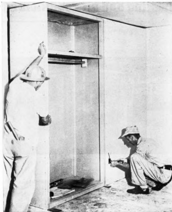
This will become more and more a familiar sight—installation of pre-assembled closet wall units
