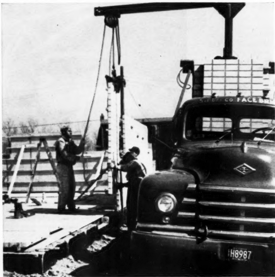
Precast brick panels being lowered into place to form steel reinforced face brick walls of a house—a technique for the future being pioneered today
