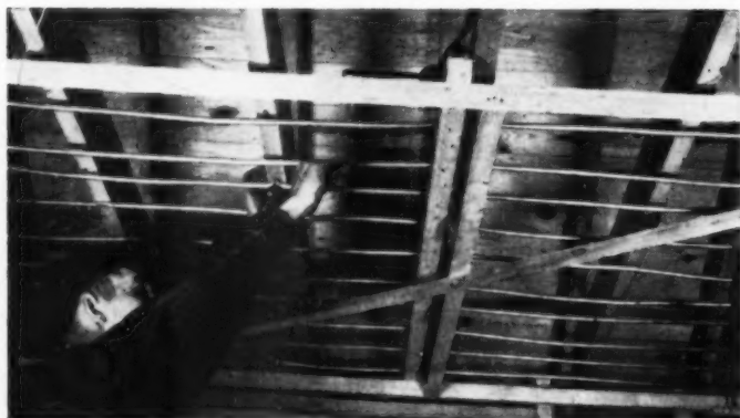
Completed coil is laid on a wood frame. The frame can be lifted easily to the ceiling where it is temporarily wired to the joists. Sufficient straps or hooks are nailed to the joists to permit the frame to be removed. The remainder of the supports then are attached
