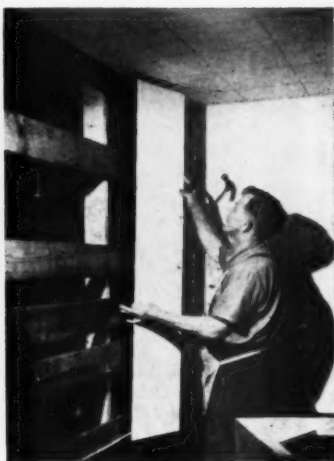
Insulation board plank was used for the walls, tile for the ceiling
