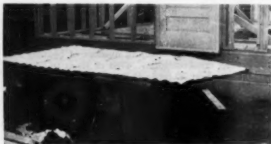
Sheathing panel looks like this after insulation has been stapled in place
