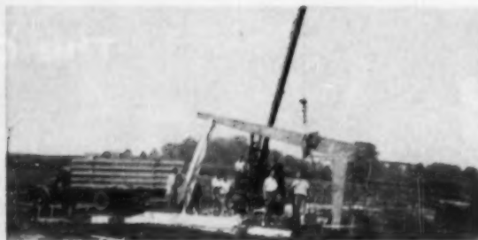
Crane and four men raised the entire concrete bent structural system and the roof slabs in 12 hours. Others shown in the photograph are VIP's
