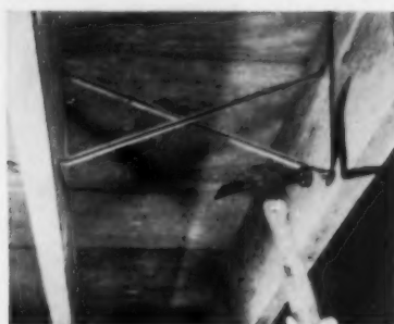
AB15311—STEEL BRIDGING —Sta-Tite, Inc., Dept. AB, 4020 N. Port Washington Ave., Milwaukee 12, Wis. Looking up at an installation of Sta-Tite bridging as the lower end of the second brace is being secured. Any small nail may be used because the flange alone secures the brace. The flanged-grips and ample bearing surfaces distribute the load independently of the nail's. Made in all sizes.
