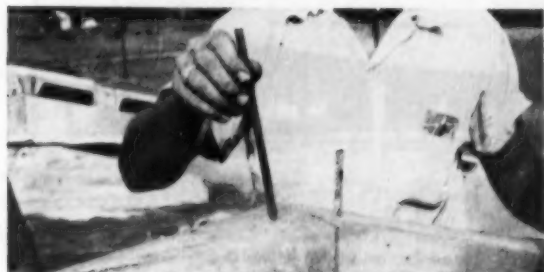
Drift pins dropped through pre-cast holes tie the bents together. Complete bent weighs 32,000 pounds and is engineered for 30 pound roof load
