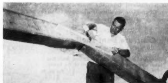
Warren installs temporary brace to provide nailing surface for temporary 2x4 spacer. Bents are cast of lightweight concrete, 100 lbs. per cu. ft. with 500 lb. p.s.i.
