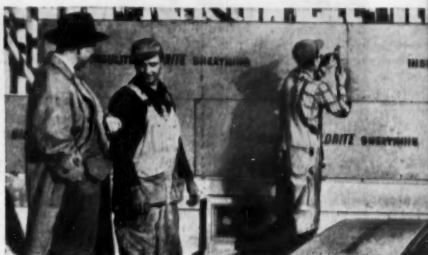
Crew follows and completes nailing. Using this system Weter's crew regularly sheaths a 1100 sq. ft. job in less than seven man hours. Bildrite goes on fast. It can cut your sheathing time as much as 43% compared with wood.
