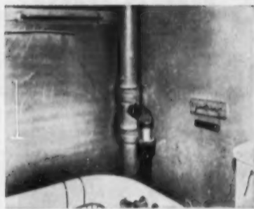
AB15332 — CAST IRON FOR SOIL PIPE —Woodward Iron Co., Dept. AB, Woodward, Ala. After 118 years of service, this 4-in. cast iron sewer stack is still in use in the oldest house in Chicago, and is as good as new. The pipe was installed in 1836. The Woodward Iron Co. furnishes many foundries with the iron from which much of the nation's cast iron soil pipe is made.
