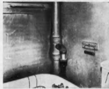
AB15332 — CAST IRON FOR SOIL PIPE —Woodward Iron Co., Dept. AB, Woodward, Ala. After 118 years of service, this 4-in. cast iron sewer stack is still in use in the oldest house in Chicago, and is as good as new. The pipe was installed in 1836. The Woodward Iron Co. furnishes many foundries with the iron from which much of the nation's cast iron soil pipe is made.
