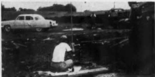
Concrete footings, 24x24x12, are spaced every 10'8" on center along building's perimeter. Bents are anchored to footing with heavy bolts
