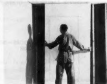
AB15045—NEW WALL GOES UP FAST—HILTON, BOOTH 4 —The Celotex Corporation, Dept. AB, 120 So. LaSalle St., Chicago 3, Ill. One of the quickest ways to finish a wall for a new room is to use materials made up in large sections. Here, a 4x8 Celotex Building Board is put in place, covering large area from floor to ceiling, is made of cane fiber. Board builds, decorates, insulates. On ceiling: Celotex Tile Board.
