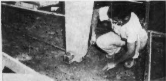
Workman tightens tie rod connecting bottoms of the bents. This relieves thrust on footing and anchor bolts. Footing takes only vertical load
