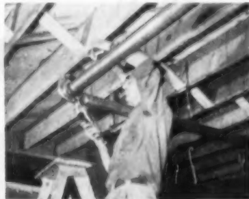
AB15047—COPPER SANITARY DRAINAGE SYSTEMS — HILTON, BOOTHS 145-146 —The American Brass Company, Dept. AB, 25 Broadway, New York 4, N. Y. Anaconda Type-M Copper Tubes, shown above with use of circular torch to make solder joint, are in 1\frac{1}{4} -in. and larger sizes for soil, waste, vent lines, are in hard-drawn, 20-ft. straight lengths, for assembly with cast bronze drainage fittings in elbows, tees, Y-branches, etc.
