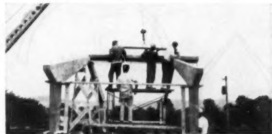
With the second bent raised, pre-cast channel roof slabs are lifted into position. Steel dowels in the bent hold the roof slabs
