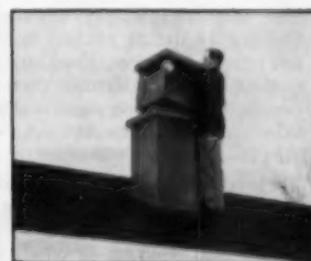
Attractive exterior chimney housing completes the installation.
