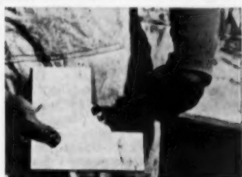
Markwa marble tile is cut to fit with the usual tile setter's tools. A tile setter's saw is used to make initial cut, clippers are used to complete it
