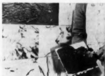
When setting marble tile with mortar, each tile is buttered and placed exactly where it belongs without twisting and then is tamped into place
