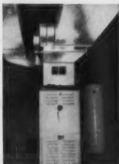
Heating Contractor for these Baltis Built Homes is Robinson Furnace Company, Chicago. This is the Robinson installed duct system of rustproof Reynolds Aluminum.
