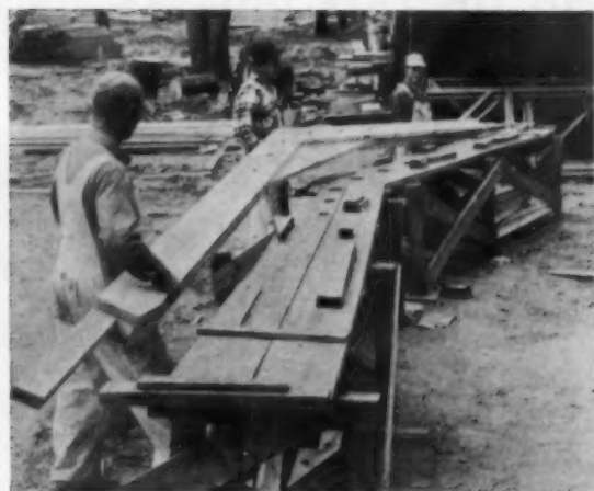
JIG TABLE for assembling trussed rafter enables two men to turn out a rafter every half hour. Pitch of 2/12 determines how blocks at ends and peak are placed. Outrigger is 2 x 4 extending 2½ feet past double rafters to form roof overhang
