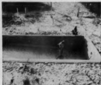
Before liner is fitted to the pool, loose earth is tamped and sloped gradually. Concrete floor is not required. Underwater lighting fixtures are in boxes below ground level
