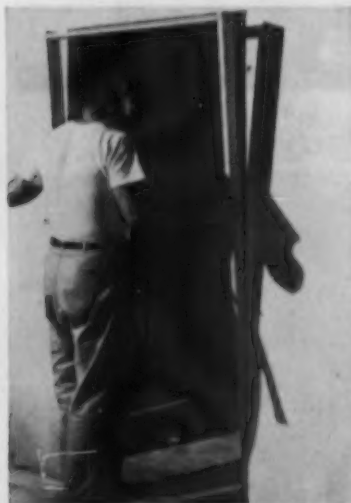
Snap-On Trim is installed after frame is placed in door opening. Saw kerfs are slots to accept trim
