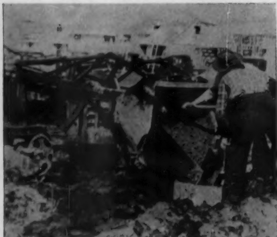
FEEDER SNOUT attached to dozer fits opening of smaller form, is used to pour batch of transit-mix concrete.
