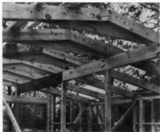
SPACED 4 FEET on center, with 13 of them to a house, trussed rafters are 24 feet in length. Nailed to these are 25-inch V-jointed, tongue and groove planks. Insulation is 2-inch fiber-glass topped with hot-mopped, coral rock surface
