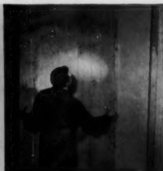
First panel is positioned by sliding one edge into place along nails driven at a predetermined joint line. Following panels are positioned by butting the edge with the un-cemented margin of the preceding panel, and swinging into place.
