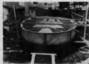
Excavation is graded accurately to conform to floor of pool. "A" frame supports pool as assembled over excavation. Plastic pipe connections are made and pool is lowered into hole
