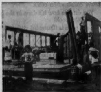
Sidewall panels were preassembled and go quickly into place as the number of small-fry sidewalk superintendents increases
