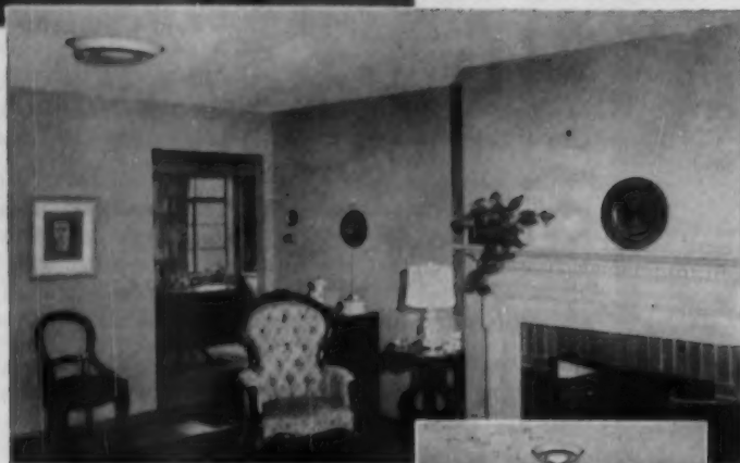
Living room has two Kno-Draft Diffusers. Air distribution system and fan-coil unit are located in attic. The condensing unit is at rear of house.
