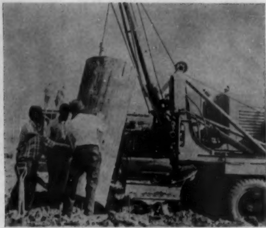
POWER WINCH drops steel form in hole, pulls it out after footing is poured. Form keeps out ground water.
