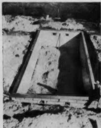
Excavation is leveled off at the maximum depth of the plastic liner and back-filled to correct slope after the walls are built. Two by 10-in. boards bolted to top of wall anchor liner
