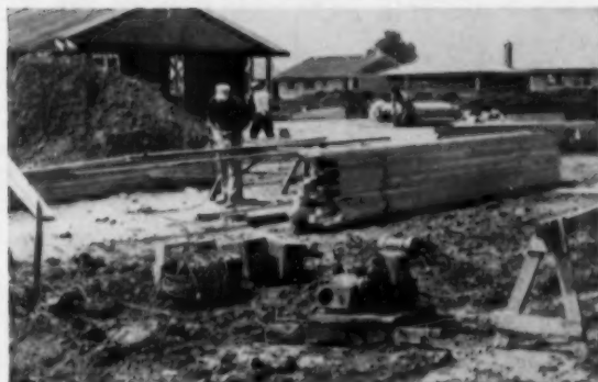
POWER HAND SAW run by a portable generator cuts joists and rafters for two buildings at pile of lumber dropped there on schedule
