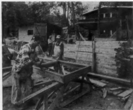
FINAL ASSEMBLY of windows consists of fitting aluminum sash in frames, then nailing on redwood surrounds. Large 16-foot frames at front of house are built in same manner—a job that many builders turn over to a millwork shop
