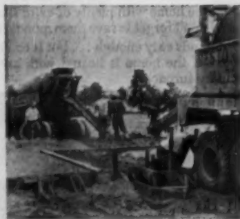
A few days before the one-day building effort, slab foundation was poured and plumbing roughed in
