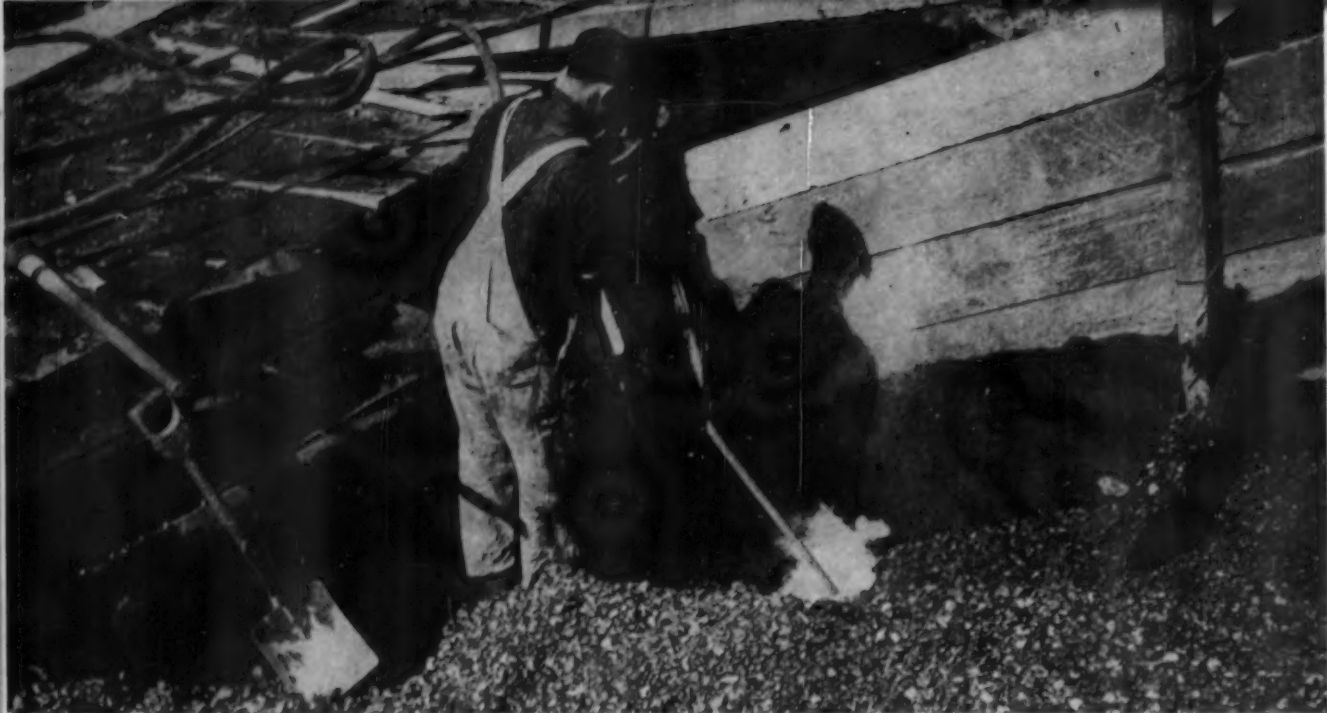
THAWING AGGREGATE with live steam jet is early morning chore when freeze hits. Just be certain that all ice and snow is removed before mixing. Raise temperature of the aggregate to 45° before adding warm water and cement.
