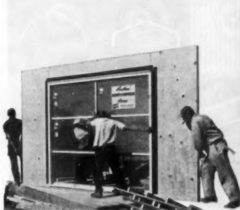
Careful Erection —Trained crews, erecting the P & H Homes quickly and efficiently, carry craftsmanship through to the last shingle.
