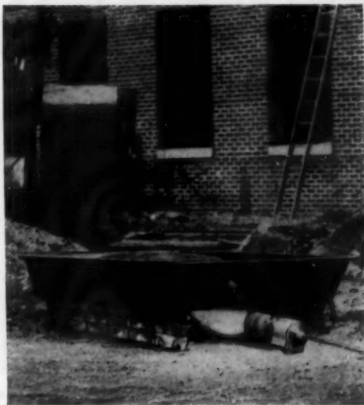
MIXING MORTAR , cement or plaster in steel box at proper temperatures is accomplished with same type of portable burner. Burner operating from 20-gallon tank at temperature of 1800°-2200°F. consumes 3 gallons per hour.
