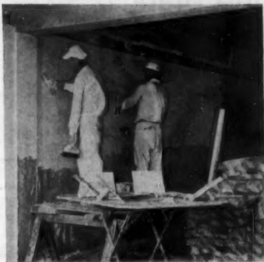
PLASTERERS PREFER to work in comfort too, but they also want plaster to dry out. Conventional heater for plasterers is salamander. Main requirement is steady heat.
