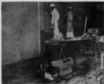
Plasterers work on the coldest days, let the heater dry plaster overnight. It leaves no oil film on plaster.
