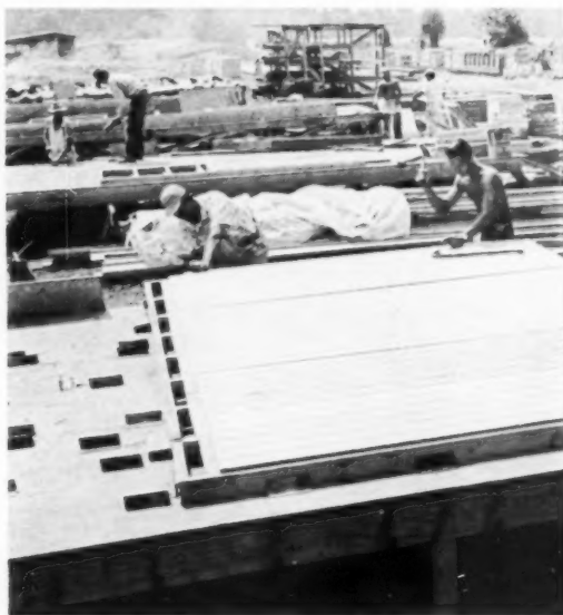
SOLID EXTERIOR WALL PANEL is built. Table can also be used for other sizes and types of panels, as shown by the additional chocks. In background are other jig tables and racks with marked bins of precut lumber.
