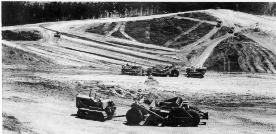
PART OF THE FLEET of massive machinery that is presently working on the Malcolm Avenue Fill in Crestmont.
