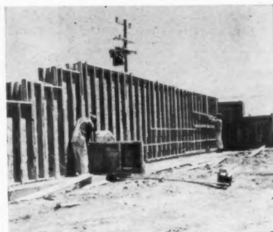
CONCRETE FORMS for combination retaining and foundation wall are set up. Diagonal braces will be set up before pouring.
