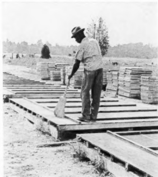
EVEN PATIOS ARE PRE-BUILT. Concrete is poured over these form tables and screeded to the top of the battens nailed on top. The result is concrete flagstones that are easy to handle, can be laid in sand without footings.
