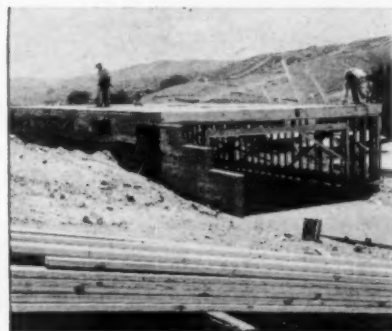
LOWER LEVEL IS FRAMED and decking for the second floor is put down. Timbers are brought pre-cut to the site.
