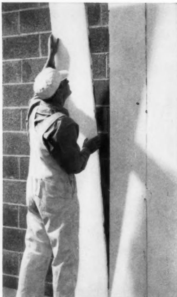
In recreation room, boards of Styrofoam are bonded to the masonry wall with Portland cement mortar, eliminating furring and lathing.
