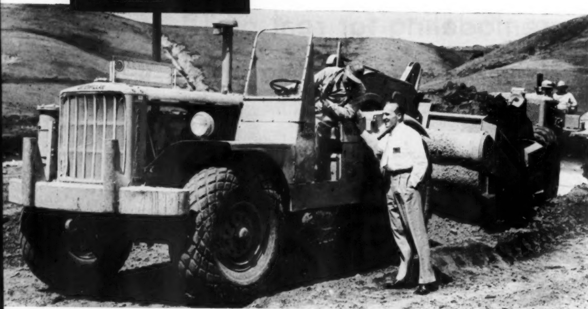
ANDY ODDSTAD is dwarfed by the tractor of a scraper rig as he talks with the operator of the machine. These
