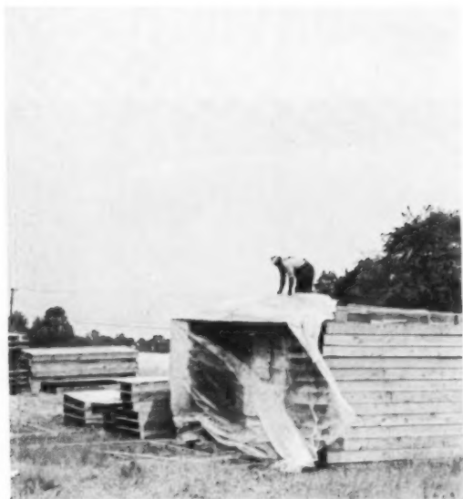
PILES OF ROOF PANELS are covered for the night with polyethylene tarpaulin. Job is quick and easy, permits every pile of panels and every table to be covered each night. Panels are easily identified through the material.
