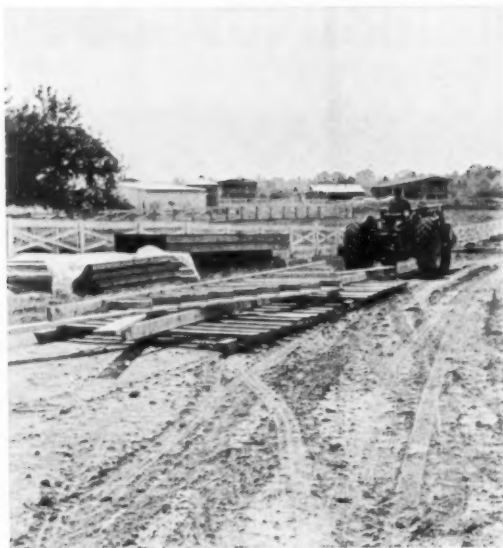
FINISHED PANELS , in this case gable ends, are loaded on skids and hauled to building sites. Skids are cheap and easy to build and repair, and do not bog down in mud. Bulldozers do the pulling when the mud gets really deep.
