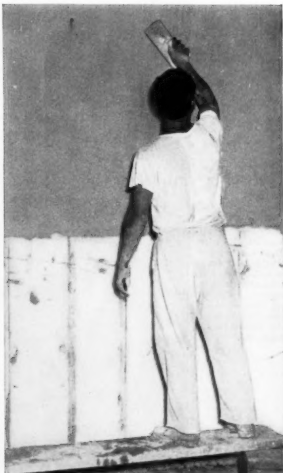
Scratch coat of plaster is then applied directly over the damp-free Styrofoam insulation.
