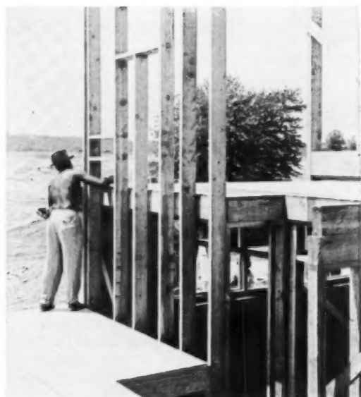
BETWEEN LEVEL FRAMING , ordinarily a major headache, is simple here. Partition of 2 x 6's balloons between all levels; instead of let-in ledgers, 2 x 4's nailed to the inside face of the partition carry the floor joists.
