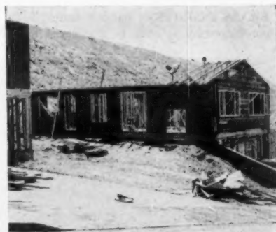
SECOND FLOOR WALLS are up and sheathed, roof trusses going up. Extra scaffolding will be necessary for finishing off.
