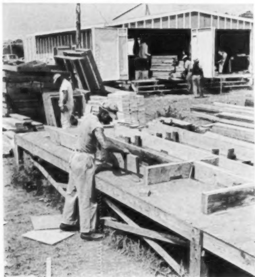
FLOOR PANELS for the deck between the levels are assembled on this table. The section under construction here is the one over the stair wells; ordinarily a tough framing job, precutting and jigs make it a simple nailing operation.
