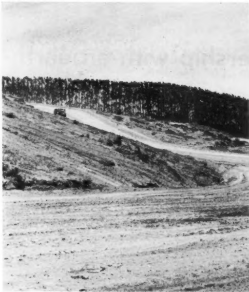
THE SHAPE OF THINGS TO COME begins to be apparent as rough grading for main streets gets under way.
