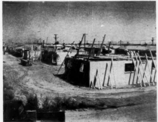
ROOF FRAMING is pre-cut and delivered on the site. The masonry blocks are stacked for easy accessibility, and are delivered to point of placement by a two-level scaffold for a minimum of waste motion by skilled masons.
