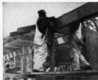
HEAVY-DUTY LUMBER is a mark of an American House. Note the large-size headers and the two by four framing members. Doors and windows are pre-fitted, pre-hung, pre-flashed.
