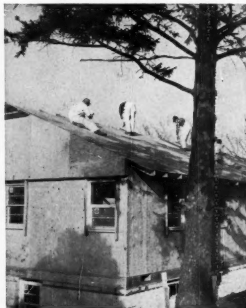
UNDER ROOF AND WEATHER-TIGHT in one working day—standard for a typical American House. Larger models usually take two days. With no weather worries, your building season is lengthened, your lumber kept dry.
