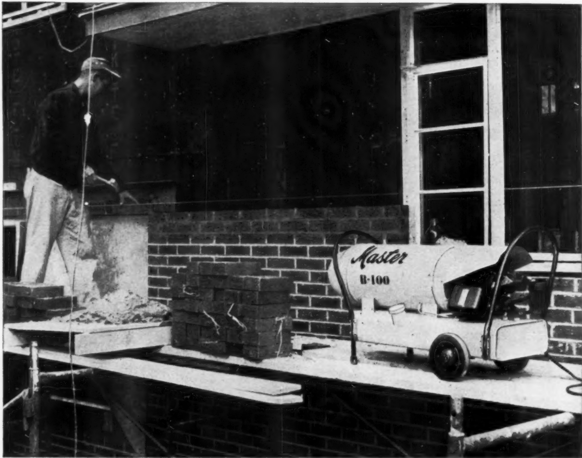
This bricklayer takes a Master B-100 heater with him on the scaffold and keeps working on the coldest days. Heater weighs only 78 lbs.
