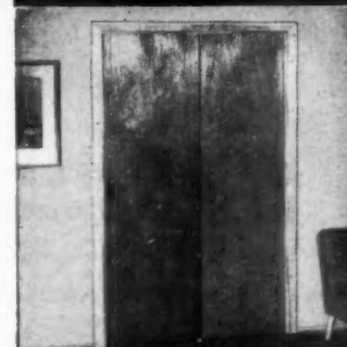
With Scottie Series 2050 hardware set to doors a neat installation is completed.
