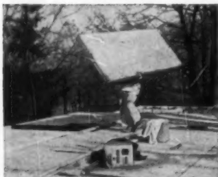
EASILY-HANDLED COMPONENTS speed construction and save labor. Accurately cut and assembled at American Houses plants, they also assure absolutely true lines throughout.
