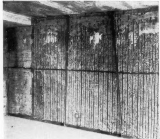
6 View of the braced side of the partition after the scratch coat has been applied to opposite side. The penetration of the plaster through the mesh provides excellent mechanical bond for the brown coat.
