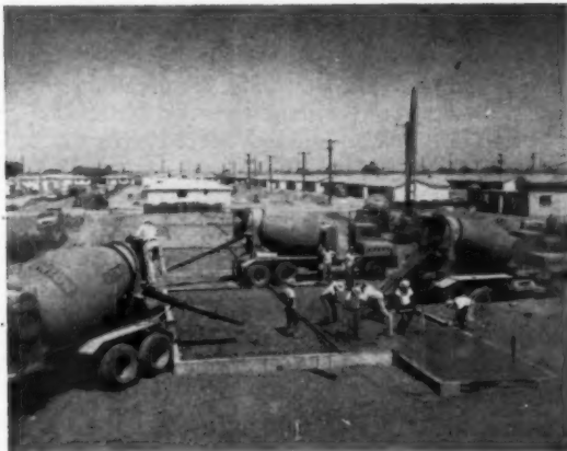
FAST SLAB POURING over concrete footings illustrates production line techniques and economies. Concrete driveway is included in the $8,000 price. Pool is put in by specialist contractor.
