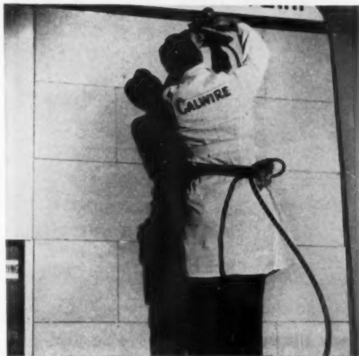
ROCK LATH IS STAPLED with this power gun, is done at incredible speed. Enough regular nails are driven to tack pieces, mark the stud positions. This man nailed off at a rate of between three and four staples a second.
