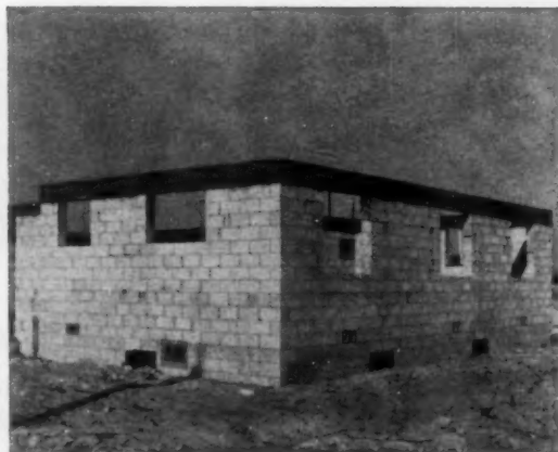
FINISHED BEAM includes the bolts shown here. A wooden header goes over them, and when it's bolted down, even a hurricane won't take the roof off.
