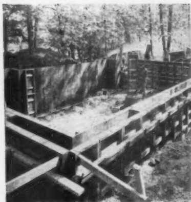
"CHAMP" Forms with cross members on 24" centers, being erected for house foundation in Skokie, Illinois. Contractor, Harding Bros., Northbrook, Illinois.
