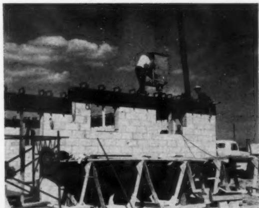
CONCRETE IS POURED into the beam forms. Combination of pre-mix truck and crane bucket permits just one man to handle the job on top of the house.
