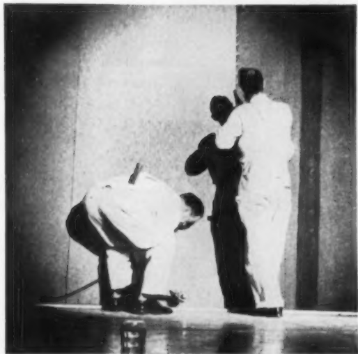
RACE BETWEEN conventional nailing and Spotnail gun is dramatic proof of the latter's great speed in applying insulating board. The gun won going away, finishing before the man with the hammer was well under way.
