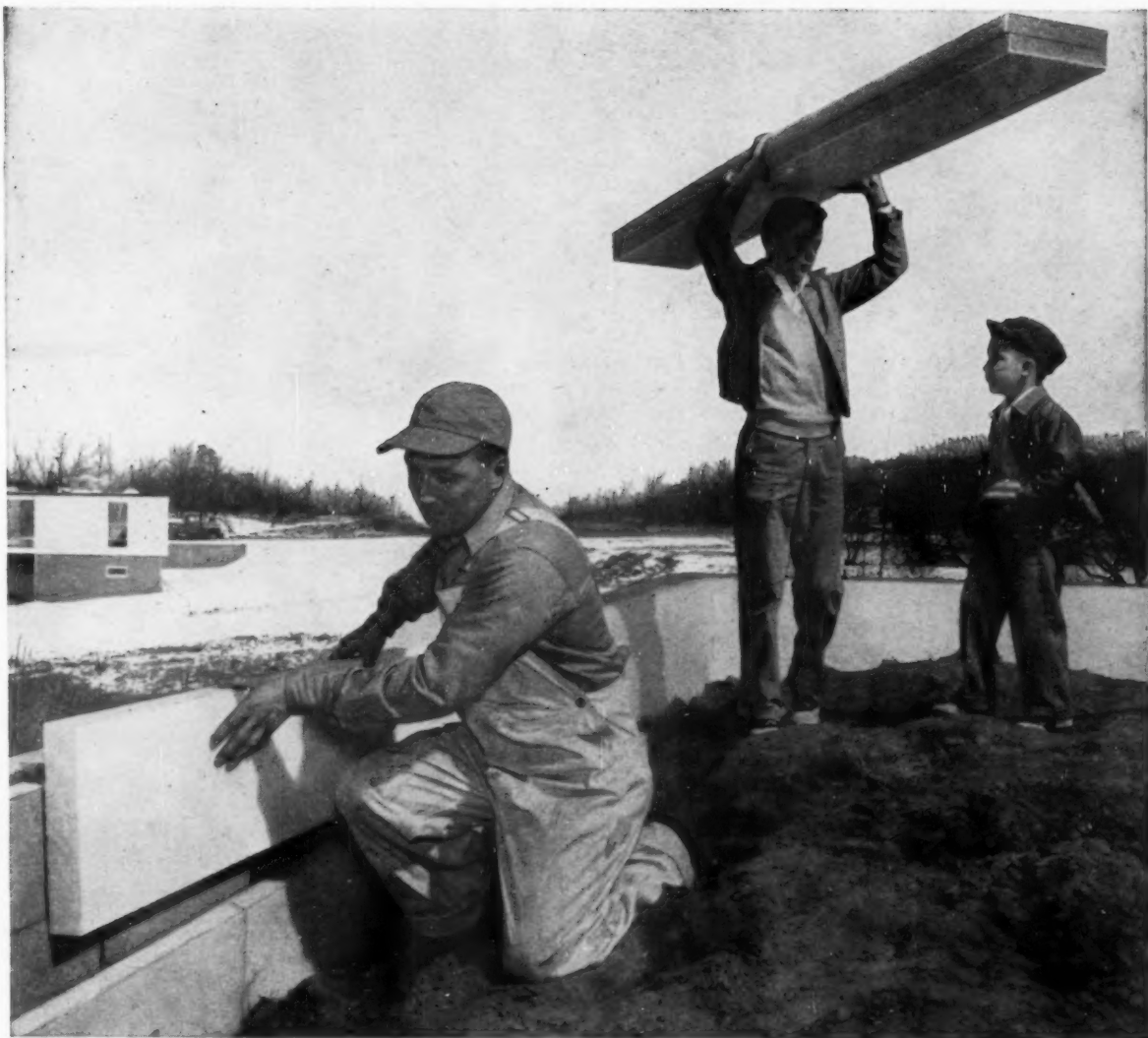
Perimeter Insulation —Wolfe & Gilchrist recommends Styrofoam for perimeter insulation in all their homes. Here Styrofoam is used in Detroit suburb to assure lifetime of warm floors and lower fuel bills.
