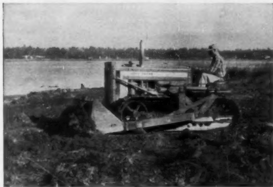
Clearing and leveling the beach is fast work for the versatile John Deere-dozer team. At times the outfit works in two to three feet of water.
