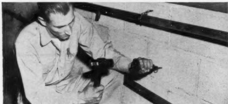
The Feldman Bros. Co., steamfitters, use a chain held by SHURE-SET wire loop fasteners, to support radiators. There's no drilling necessary.
