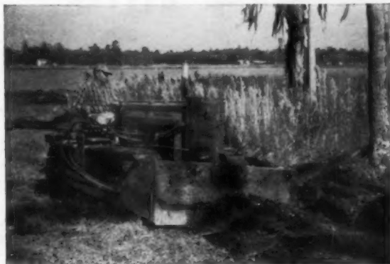
To move unwanted trees, Mr. Harvey uses one corner of the tilting dozer blade to loosen earth and cut lateral roots.
