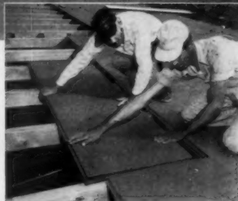
Tri-Dek is nailed to rafters. Finish roofing is applied over it. Job's done!
