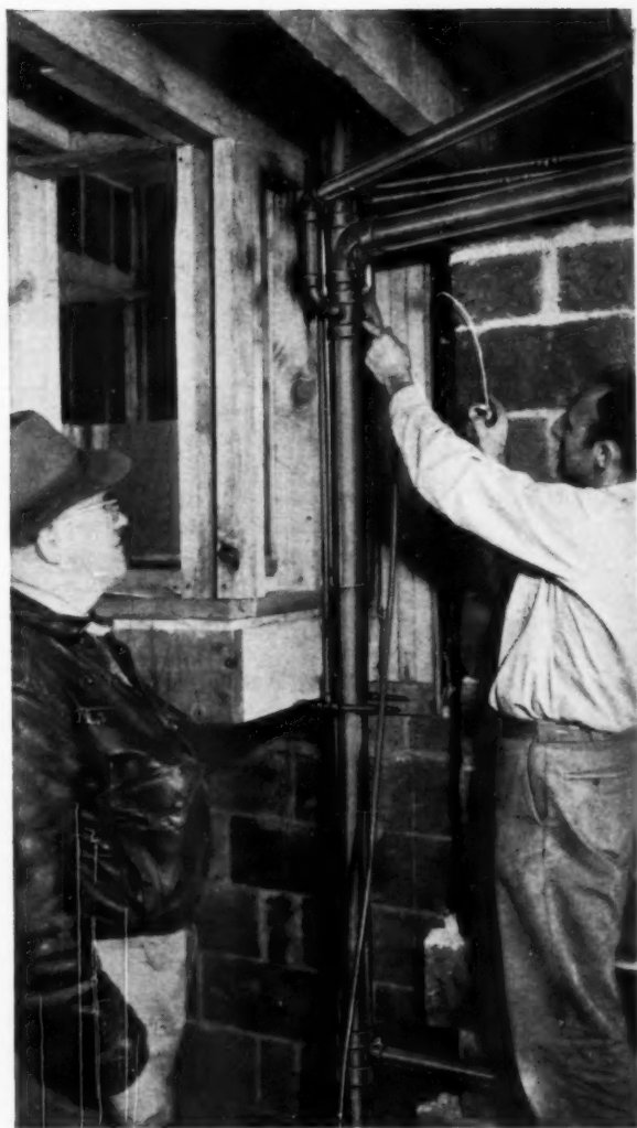
J. L. FITZPATRICK of J. L. Fitzpatrick & Sons, Jenkintown, Penna., plumbing contractor for Rockledge Homes development, watches journeyman Sam Duper, Jr., connect a 3-inch copper tube soil line from bathroom to the stack. Anaconda Tube for the development was supplied by Fleck Company, Elkins Park, Penna., plumbing supply wholesaler.
