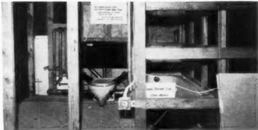
NEW BATHROOM fixtures now permit above-the-slab plumbing, but many outdated codes say: "Absolutely no."
