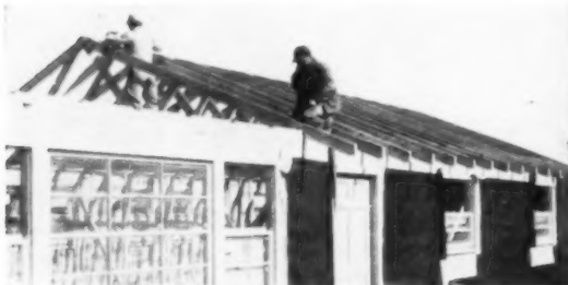
ROOF TRUSSES are outlawed completely in some areas. Here, they're on 24" centers—also blocked by old codes.
