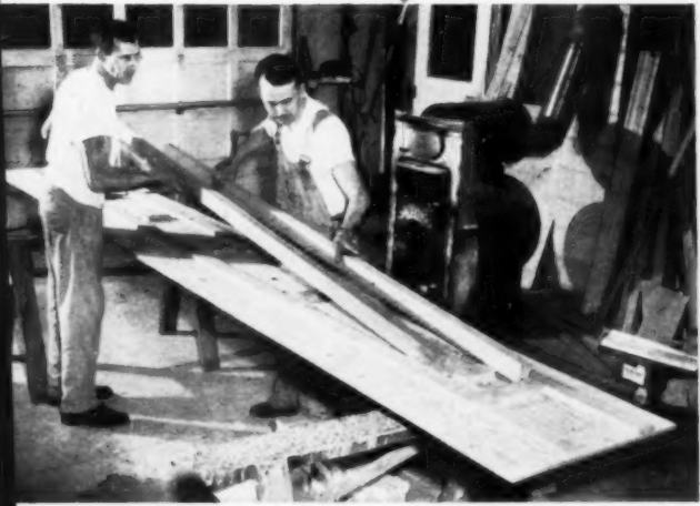
BUILDER uses simple jig set-up to construct box beams. For a larger operation (100 homes) some sort of press set-up would be needed. Douglas Fir Plywood Assn. is coming out soon with booklet showing best method.
