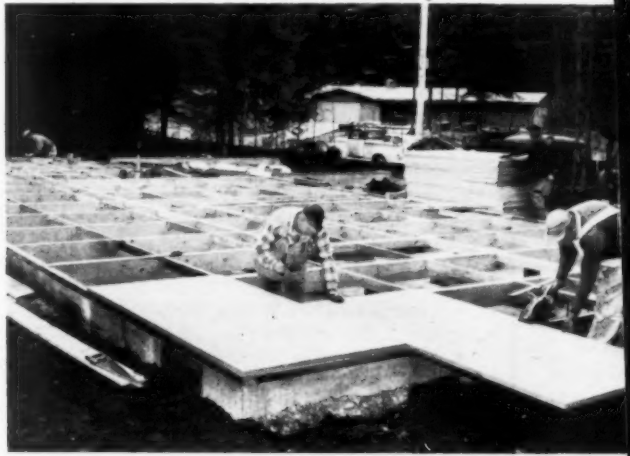
WORKMAN can be seen nailing down first sheet of 1 1/8" plywood sub-floor over box beams. Structural system consists of beams which run 4' O.C. with 2x4's attached by metal anchors which are also placed 4' O.C.
