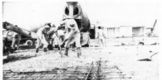
REINFORCED grade-beam slabs could go down fast; eliminate cost of digging and setting spread footings.
