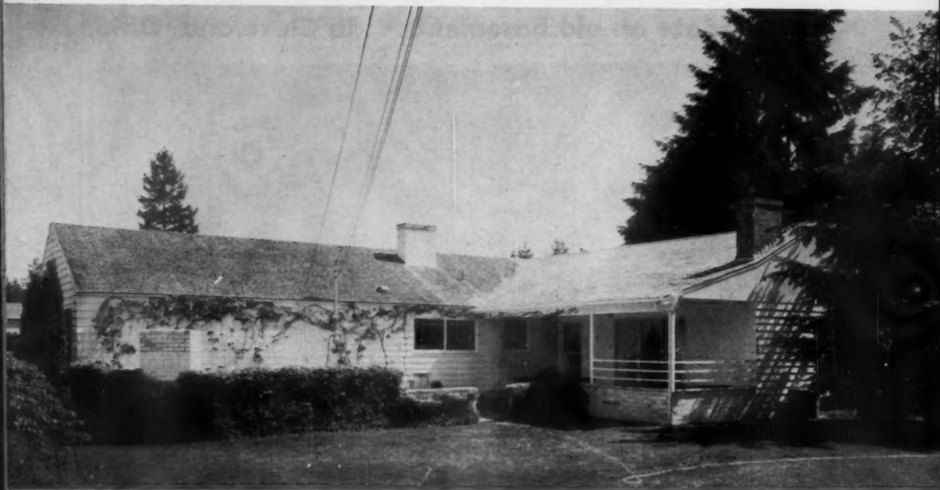
AFTER: A 24'5" x 9'8" porch on new wing leads out to existing patio. Porch decking is 2 x 4 redwood.
