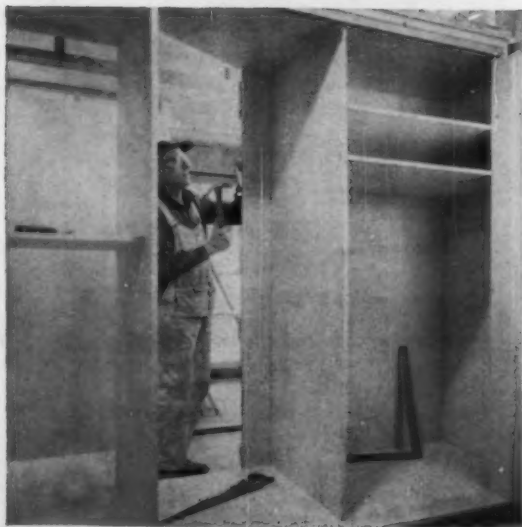
INTERIOR paneling of new room is \frac{3}{8} " fir plywood, "PlyPanel." It was placed directly on the studs. Built-in wardrobes and cabinets were of fir plywood. Material was easy to work, provided smooth painting surface.
