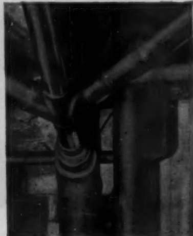
8" soil stack and 6" vent in 43-story office building. Space-saving, easily installed solder-joint fittings are a big advantage in large work like this.
