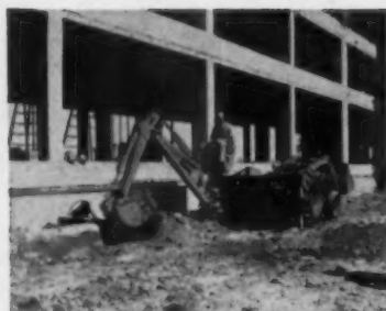
The Davis 210 Backhoe on a Work Bull 202—the only machine in the world that can dig flush alongside a wall.
