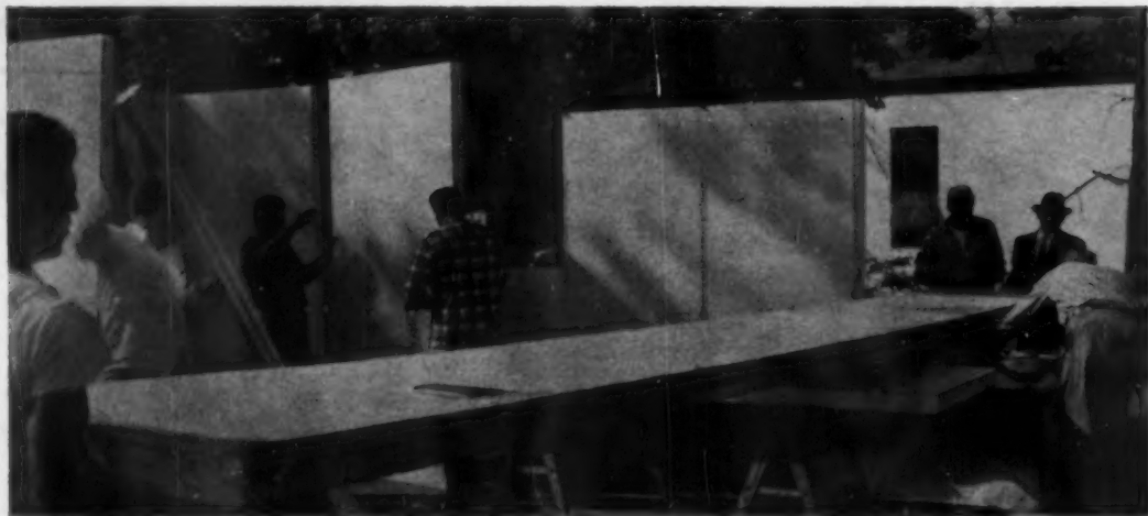
ROOF PANEL will span 24 feet. Rails, glued to edge, form T and G joint. Plastic tape seals joints on top.
