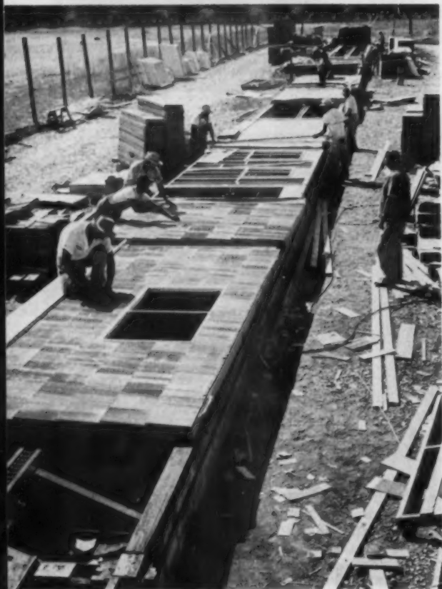
ASSEMBLY LINE speeds up "manufacture" of exterior walls. Each man does a different job. Production begins at the far end of the line. By the time the panel reaches the last man, only cedar shakes have to be nailed on.
