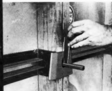
Tie-rod pin is inserted and tapped with hammer to secure tie-rod which automatically gives desired wall thickness.
