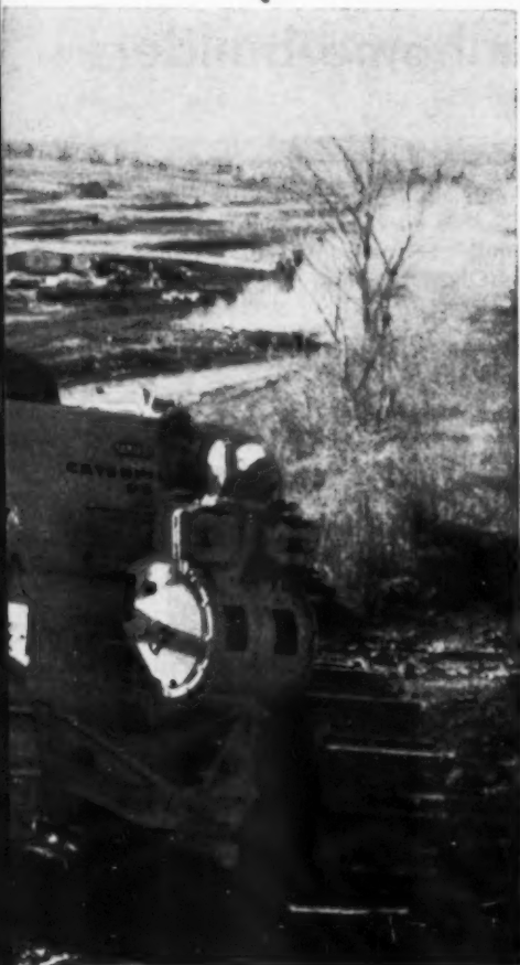
◀ FIRST THE CUT —Catepillar D8 push loads a Cat DW 15 scraper taking a 15-yd. cut of earth from hilltop. Scraper then hauls earth to base.
