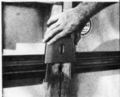
Clamp easily slips over metal-wedge ears of adjacent forms. One blow with hammer locks clamp.
