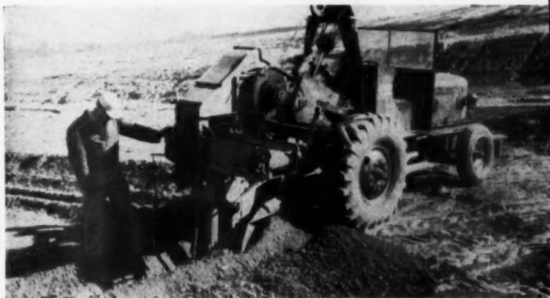
FINALLY THE TRENCHES —Barber-Greene pneumatic trencher fitted with special attachment digs foundation trench and bells out footing.
