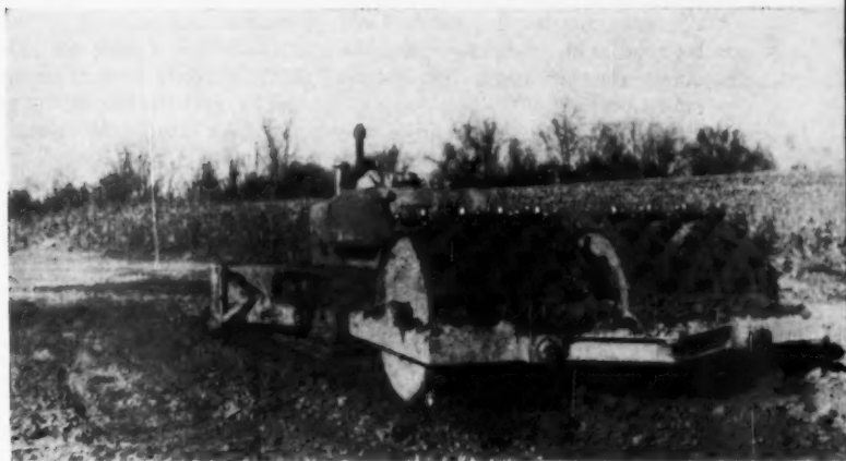
NEXT THE COMPACTION —Cat D8 tractor pulls pair of Tamco sheepfoot rollers over 6-in. lift to bring fill to specified density.
