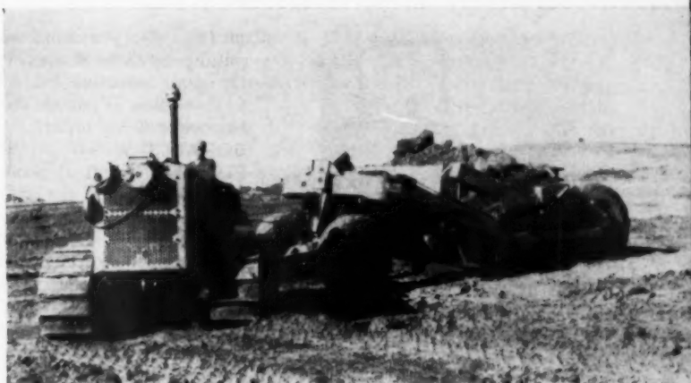
THEN THE FILL —Scraper deposits fill taken from hilltop in 6-in. lift at low areas of subdivision. Method balances high and low contours.
