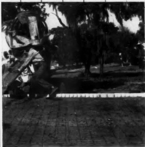
▲ ONE CREW CONCRETES —Transit-mix truck pours concrete over wire mesh reinforcing to start slab for one house. Plumbing has already been placed and covered with fill.
