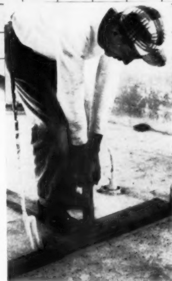
▲ ANOTHER FRAMES —Workman wielding Ingersoll-Rand powder actuated nailer toenails cedar plate into slab. Top-grade cedar goes throughout this quality-built house.
