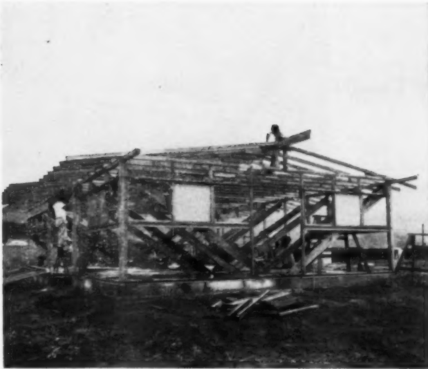
TRUSSES are set on top of completed sidewall frames. Roof goes on before siding, since rain (and Hawaii has lots of it) would stain the unfinished redwood skin.
