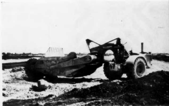
SCRAPER SPREADS FILL IN 6-IN. LIFTS —Caterpillar DW21 self-propelled scraper carries fill from borrow area and deposits it in small lifts along trench over which builder will put up row of houses.
