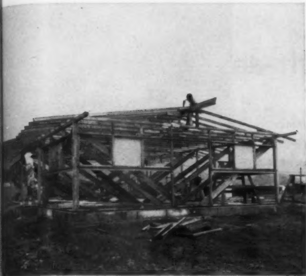
TRUSSES are set on top of completed sidewall frames. Roof goes on before siding, since rain (and Hawaii has lots of it) would stain the unfinished redwood skin.
