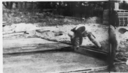
SAND BED 2 in. thick is struck off to receive floor panels. Sand is spread on a 4½ in. layer of fine gravel. Idea is to make slab winter-proof; only the
