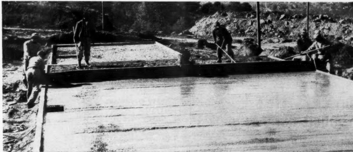
1. Making first pass with 24 ft. 8 in. Stow vibrating screed. 16 man hours per slab saved by Major Building Co.
