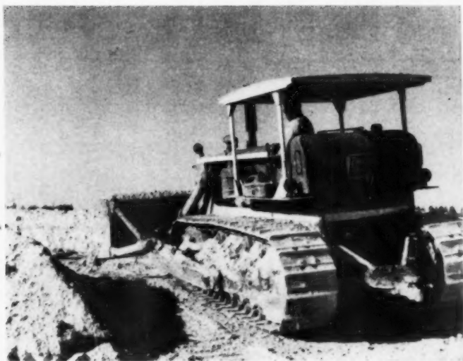
BULLDOZER READIES BASE FOR EMBANKMENT —Caterpillar D8 fitted with bulldozer blade trims bedrock to ready it for embankment construction. Embankment will be built up 5 ft. wider than houses.
