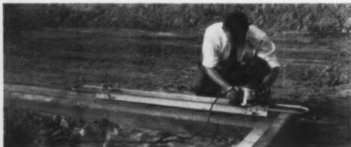
ACCURATE SILL LEVEL is necessary for proper alignment of wall panels. This device guides router, which cuts sill to right line. Bottom 2x4 is shot to foundation wall; top, or "sacrificial" sill, is nailed with aluminum nails, which router can cut. After the cut is made, top sill is spiked into place.
