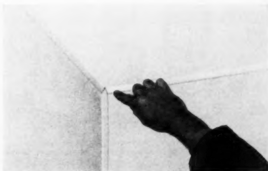
FINISHED WALL looks like this. In a model house, where hundreds of people went through, only two or three noticed and commented on unusual appearance of bevel corners.
