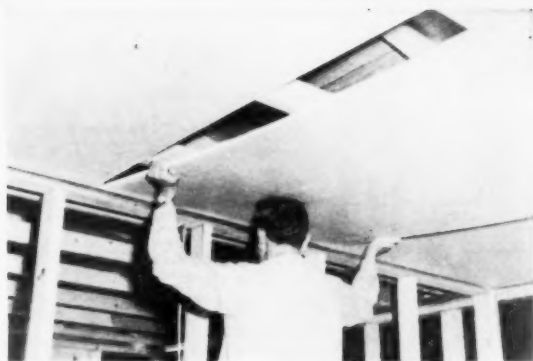
CEILING BOARD is pushed into Steelfast strip. If joists are uneven, strip is set at lowest point, and the first nailing of board to joist is made 24 in. away from the corner.
