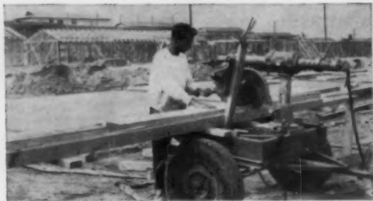
2 Headers are precut with radial saw. Key to speed of entire framing operation is in utilization of right power tool for each operation.
