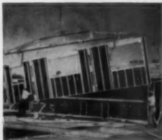
INSULATION BOARD sheathing is tied to firm's success; they make 300 lineal ft. of walls daily.
