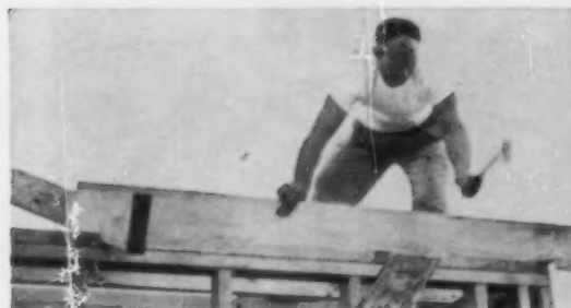
9 Two-man crew sets roof joists. Elapsed time on this phase of the operation is five man-hours. Power tools make the difference.
