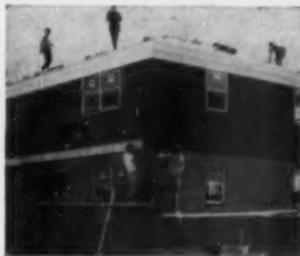
APARTMENTS will be brick-veneer up to 2nd floor; shakes will finish job. Breckwood built 250 homes in 1959.
