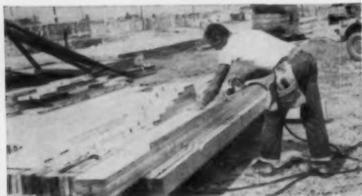
1 Rafters are precut while the lumber is still piled off-slab. Aim of the entire operation is to minimize movement of men and materials.
