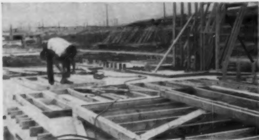
4 Panels are nailed together on slab. Headers, studs, bracing, have all been precut and stacked for assembly. One man specializes in this operation.
