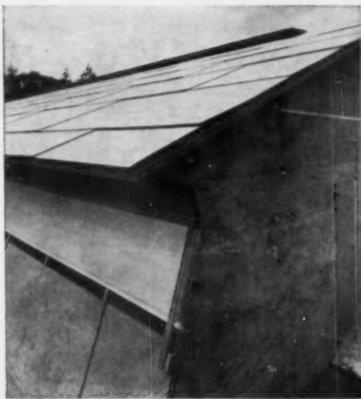
OUTSIDE WALLS get covering of exterior grade fir plywood. Roof sheathing (also plywood) may be covered with roll roofing, or with shingles of wood or asphalt.
