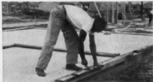
3 Layout man marks off sill plate for placement of studs. One man, using a template, concentrates solely on this operation, achieves terrific speed.
