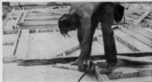
6 Raiser cuts dado for placement of 1"x6" brace. Each workman is skilled with the particular tools required for his phase of the operation.
