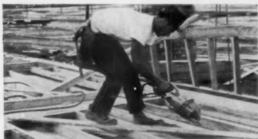
7 Shot of dado cutting along panel studs gives some indication of speed and skill achieved by carpenters. Observers liken them to Keystone Cops.
