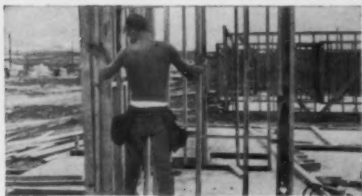
5 Raiser places completed wall sections on preset bolts. Entire raising operation—framing, setting, bracing—takes only eight man-hours.
