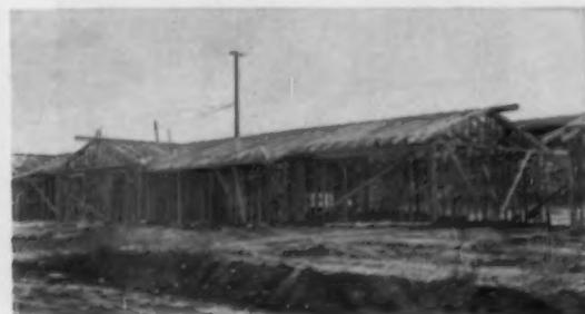
10 Entire 1,400-sq.-ft. house is framed out in 25 man-hours, plus two man-hours for cleanup. Total framing crew consists of nine men.
