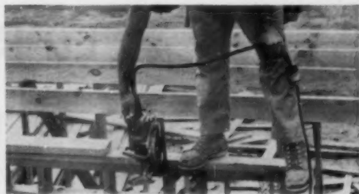
8 Two-man crew sets roof pitch supports, cut and nail into place—total man-hours, five. Roof framing is most complex phase—takes ten man-hours.
