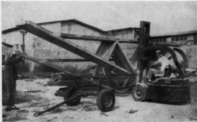
MATERIALS HANDLING devices add greatly to component building costs. Fett builds on 18-day cycle; claims scheduling is the real secret of component construction.
