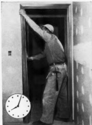
8:03 a.m. Now strike jamb is placed into starting position and rotated to vertical position. Beveled profile of E-Z Frame harmonizes well with contemporary decor.
