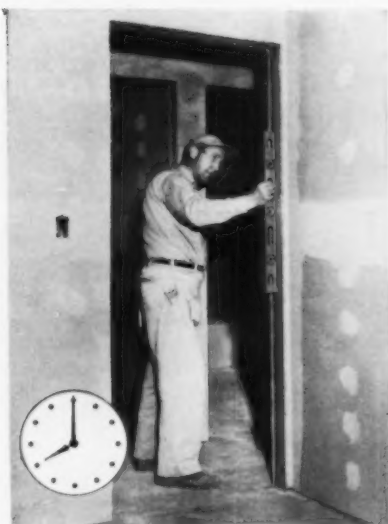
8:00 a.m. You are about to view a new, cost-saving, one man "K-D" frame installation for wood doors using Amweld Steel E-Z Frames. E-Z Frames are installed OVER 1/2" drywall! First, the wood stud is checked for plumb.
