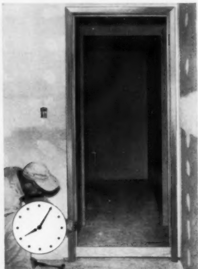
8:05 a.m. Base anchors at bottom of jambs are nailed and the strike plate and rubber bumpers installed. No nail holes to fill . . . anchors covered by base molding.
