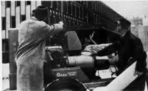
On-site power for construction tools, lighting in areas beyond mainline service.
