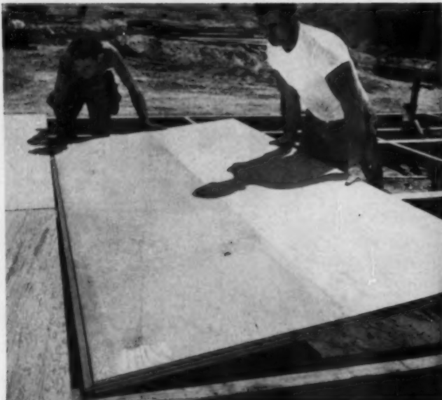
SPEEDY —Workmen fit tongue and groove subfloor panel into place on a California housing job. Method developed by Doug-
