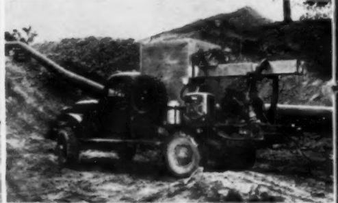
Portable power for pipeline X-Ray equipment, lights, tools and communications.
