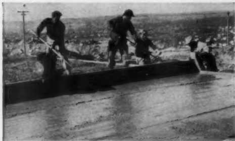
2. 4-inch slump concrete is screeded. Note the termite shield at edge of slab.
