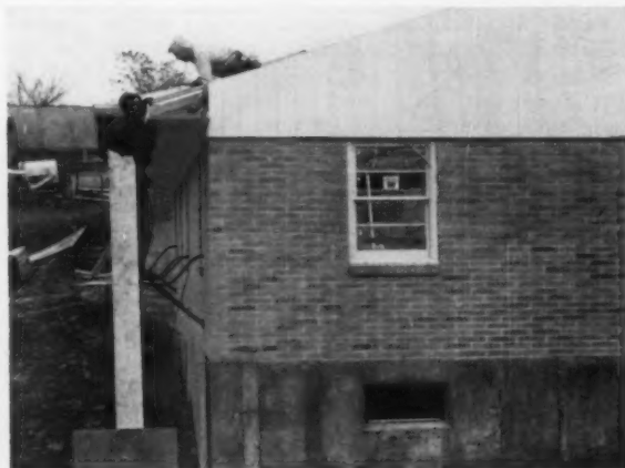
TO INSTALL SOFFIT , top is nailed into the trim board. Gable ends are prefabricated and primed—ready for finish coats. McFarling uses fork lift equipment to position gables for nailing.
