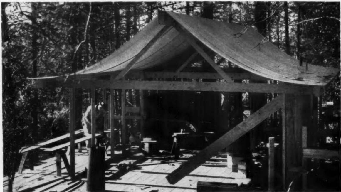
TEST HOUSE shows plywood panels formed as curved roof between roof beam and wall plates, giving design a Far Eastern look.
