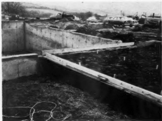
FILL at right is for garage slab. Concrete wall at angle is actually reinforced concrete beam. To cut costs, driveway, sidewalk are poured at same time garage slab goes in.
