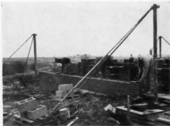
STORY POLES speed and assure perfect job. SCR masonry process is adapted to bricklaying inside. The SCR brick is all laid from inside; it's palletized, set on deck by lift.
