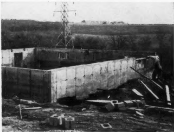
FOUNDATION WALL goes in next; and house is ready for floor system. Block wall is garage foundation (plan). Reason for switch is grades vary; it saves to go just to frost line.
