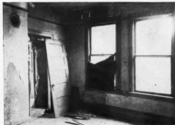
Before: Dilapidated dining room
