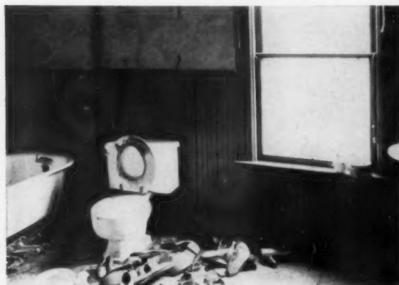
Before: Bathroom adequate, but antiquated
