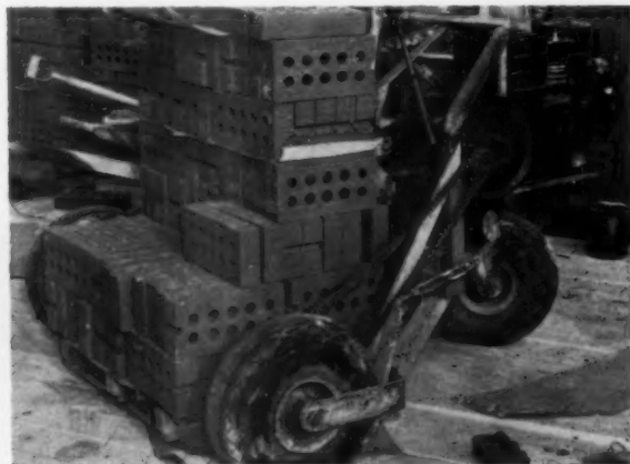
BRICK BUGGY is another McFarling invention. Crews use it to distribute palletized SCR brick around deck. Machine cost about $1,000 to make, saves roughly $35 per house in labor time.
