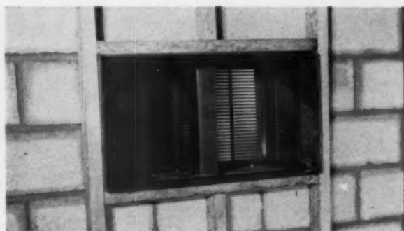
INTERIOR FRAMING is also simplified. Only one stud needs cutting, and addition of two single headers forms a perfect frame.
