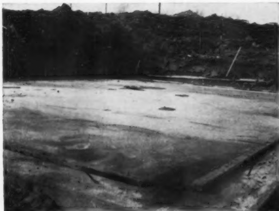
BASEMENT FLOOR is placed before basement walls, saves steps in placing the slab and footing together. To date, there has been no leakage. Trick also gives surface for forms.
