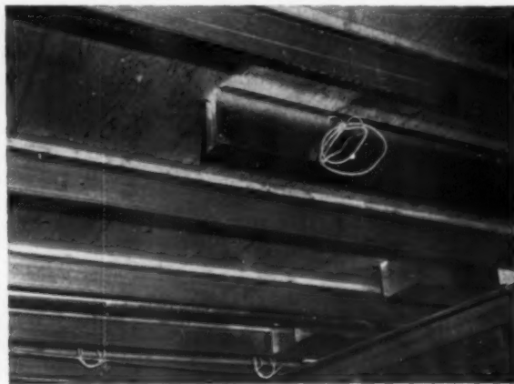
BASEMENT CEILING is fabricated with junior beams and 2-4-1. Big advantage of placing basement floor first is that it facilitates use of large screed and finishing machines.
