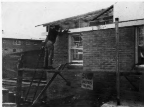
PRIMED TRIM BOARD is installed to receive prefab soffit, which is made up in 8' sections and primed against the weather. Note use of scaffold brackets, which speed jobs with safety.
