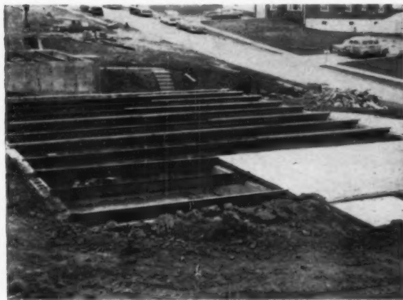
POCKETS FOR BEAMS in foundation walls are handled conventionally. Junior beams are used: Builder has had shrinkage problem with wood joists, which caused base separation.
