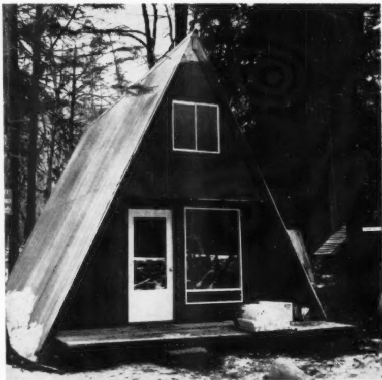
It took only six hours to erect complete shell of this house
