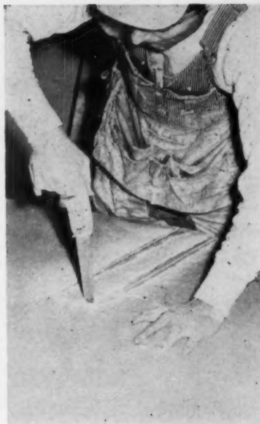
CUTTING PANELS for beams and doorways is easy with hand or power saws.
