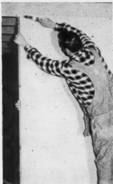
PLATES are nailed to floor and ceiling, after which panels are nailed to plates.
