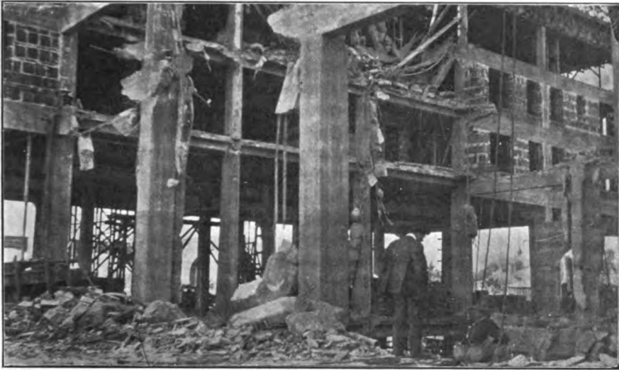
View Showing Condition of the Basement after the collapse.
