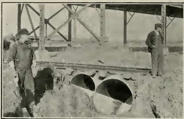
Fig. 1. Showing Ingot Iron Culverts, one 36 inch and the other 46 inch Beneath Railroad Ties
