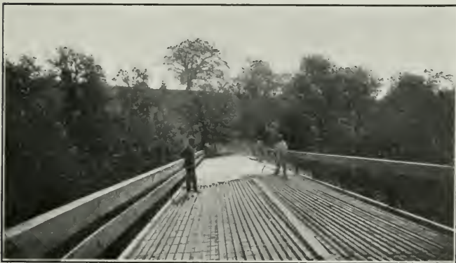
Fig. 2, Showing Timbers Placed Lengthwise of the Bridge, and Concrete Wearing Surface on Deck Span
