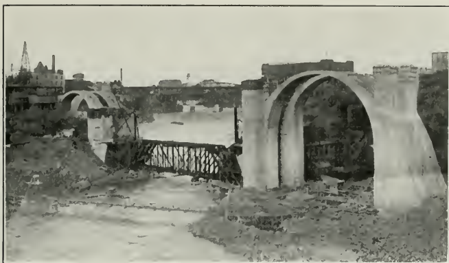
Fig. 1 View Showing Spokane Arch With Steel Trusses in Place to Receive 281-Foot Timber Center
