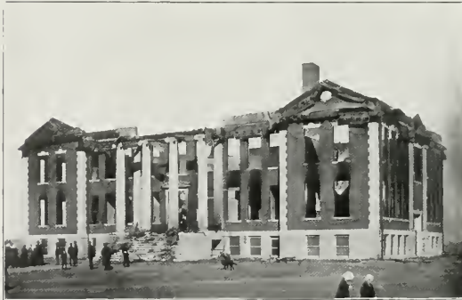
The Same Building After a Fire on February 4. Absence of Fireproof Floors was Responsible for the Extensive Damage. A few Thousand Dollars Spent for Concrete or Hollow Tile Fireproofing Would Have Confined the Fire to at Least One Floor, if not to a Single Room.
