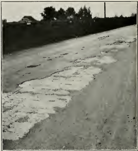
STATE ROAD NEAR SAN JOSE Showing bituminized top worn out
