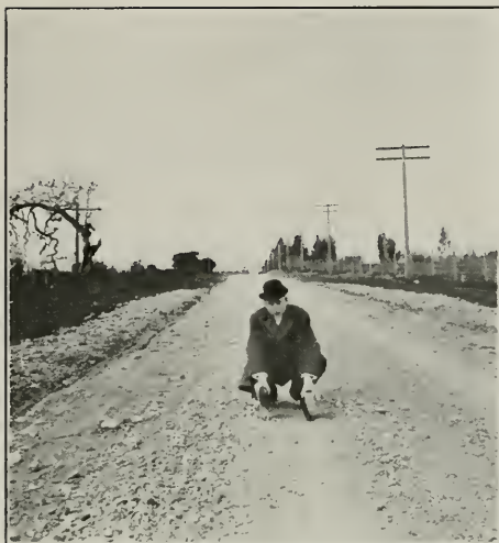
STATE ROAD NEAR HEALDSBURG Concrete torn up for about 700 feet—too thin. Photo taken March 1, 1914
