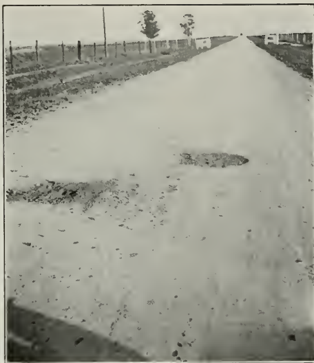
OILED MACADAM ROAD NEAR MARYSVILLE Surface breaking away
