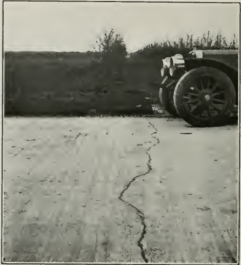
STATE ROAD NEAR SAN JOSE Shrinkage crack
