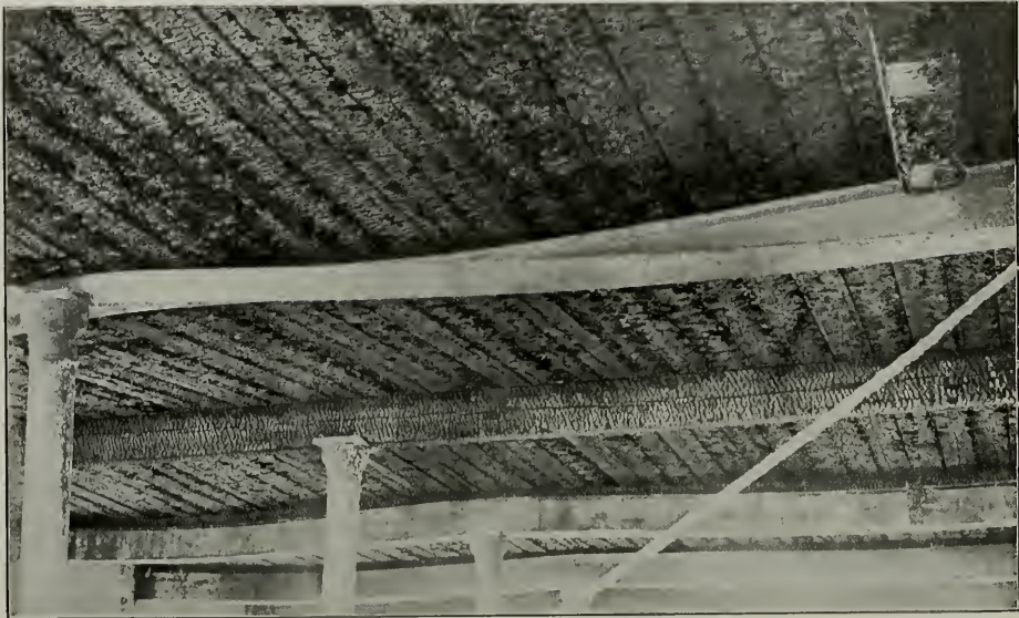
Wooden Timber vs. Unprotected Steel Beams. The stability of the single eight by ten inch wooden timber was not affected, although the ten inch steel beams sagged and were twisted to a degree which required rebuilding. The wooden beam was used because not enough steel had been ordered to complete the work promptly. In rebuilding, wooden beams were used throughout.
