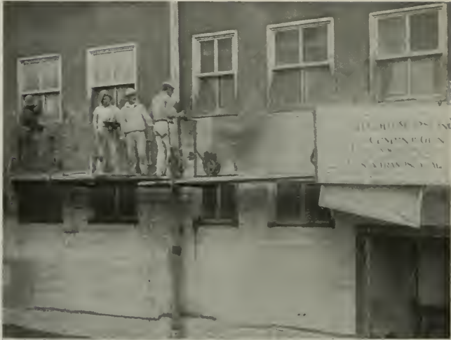
REAR WALL OF HALE DEPARTMENT STORE, SAN FRANCISCO, being waterproofed with the aid of the Cement Gun. Part of the west wall of this building was similarly treated several years ago and it was the only dry spot during the recent heavy rains.
