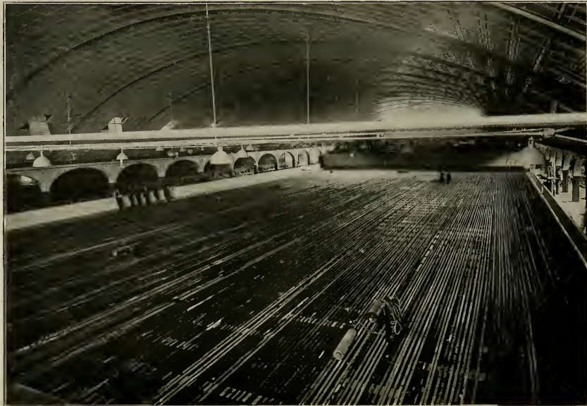
TEN AND ONE-HALF MILES OF STEEL PIPING WELDED TOGETHER FOR THE FORMATION OF AN ARTIFICIAL ICE POND
