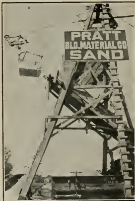
Sand Loading Plant on the Yuba River at Marysville
