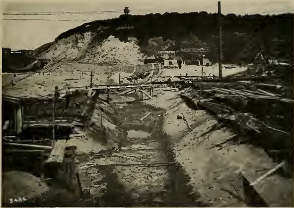
BUILDING SECTION B PREPARATORY TO PLACING H-BEAM GIRDERS. SHEET PILING IN PLACE
