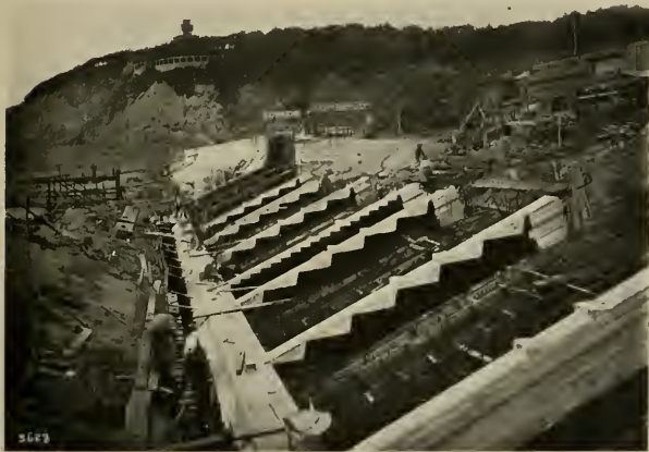
SECTION B OF ESPLANADE. H-BEAM GIRDERS AND REINFORCEMENT FOR BLEACHER SLABS IN PLACE
