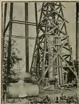
Corrugated Well Curbing being placed in municipal well at Clovis, N. M. The installation of 240 feet of 36" diameter was accomplished in twelve hours. Material was No. 14 gauge galvanized "Armo" Iron.
