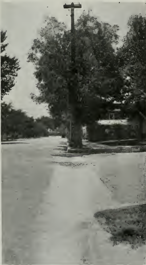
(Fig. 4) SHOWING OLD DIP ON WEST SIDE OF B AND 18TH STREETS, BAKERSFIELD. NOTE RAVELING OF CONCRETE CAUSED BY JOUNCING VEHICLES
